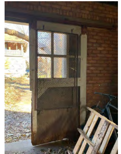
Site Photo 4, by Applicant, showing interior condition of the garage door.
