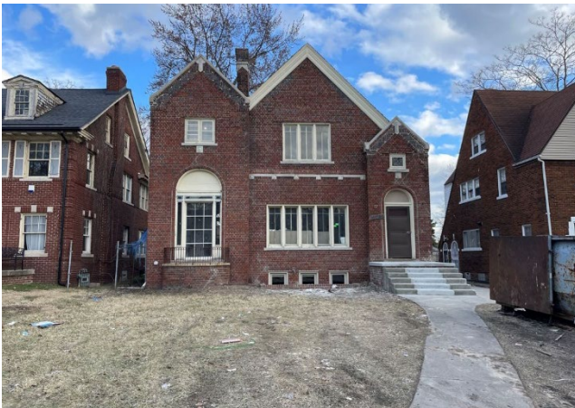
Site Photo 1, by Staff March 25, 2022: (Northwest) front elevation, showing new front porch landing and steps.
