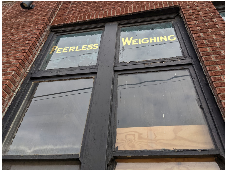
Detail view of large wood windows at first floor. Staff photo, November 2, 2021.
