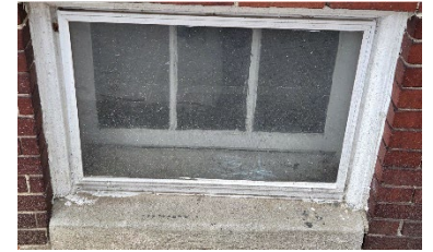
Site Photo 3, by Applicant, showing exterior condition of original basement window at 391-393 W. Grand.
