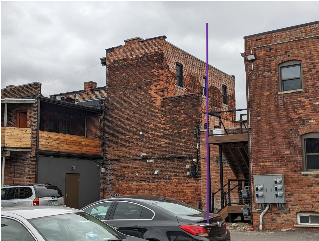
View of 3-story section at 1444 Michigan, view towards the southwest. This is the location of the proposed one-story garage addition, to be placed on 1416 Michigan (foreground). Note substantial brick repair and parapet work recently completed on the 3-story section. Structure at right is the Elizabeth Street building (not in the historic district, though it shares the same parcel). Purple line gives an approximation of the district boundary, and location of what will become the tallest element in this composition. Staff photo, April 1, 2022.
