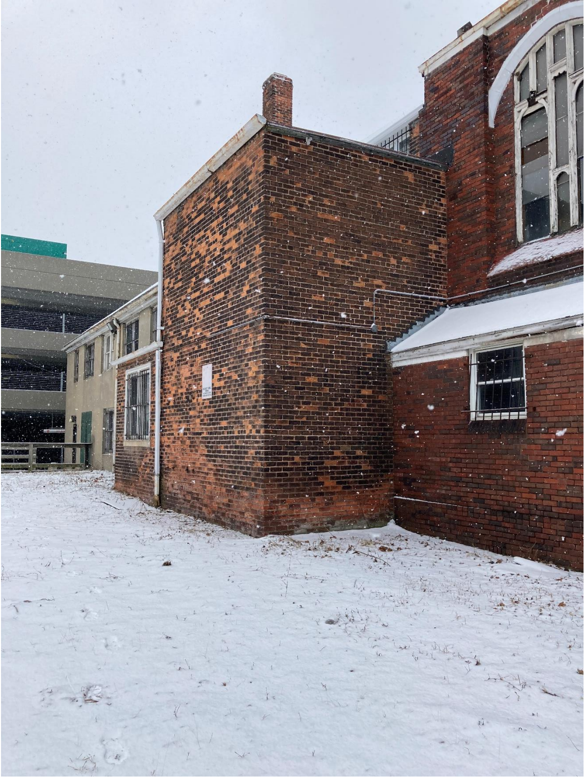
This wing will be demolished, with new wing to be built within the same footprint. The second-story portion of the new wing will be higher than the current. The existing brick will be reused to clad the new wing.
