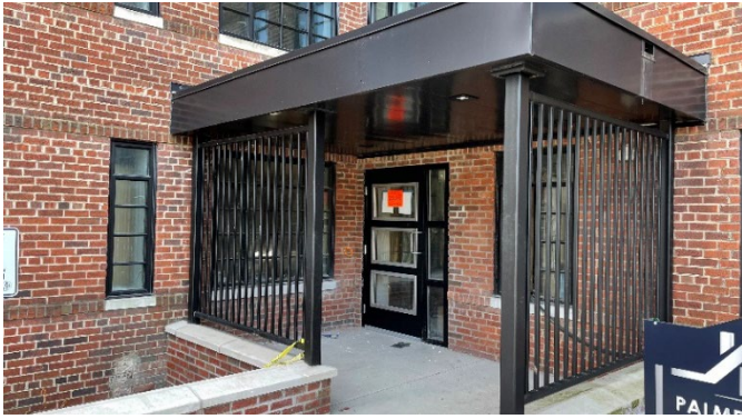
Site Photo 7, by Staff, February 24, 2022: (North) front elevation of 885 Covington showing thicker canopy and vertical panels.
