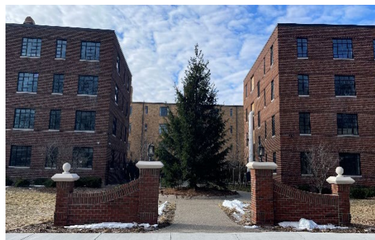
Site Photo 6 by Staff, February 24, 2022, showing new brick "wing walls", courtyard entrance, and evergreen.
