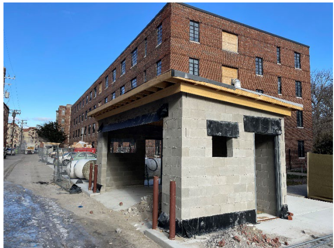
Site Photo 3, by Staff February 24, 2022: (South) between 885 & 931 Covington, showing partially built 12’x22’ trash structure. Roof and window openings will be removed to reflect architectural drawings.
