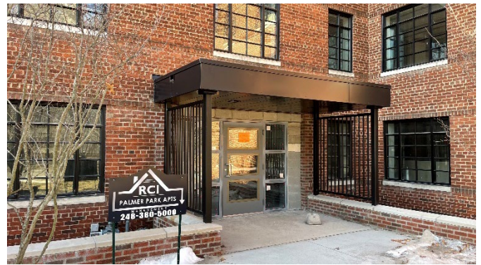
Site Photo 8, by Staff, February 24, 2022: (North) front entrance of 931 Covington showing thicker canopy and vertical panels.
