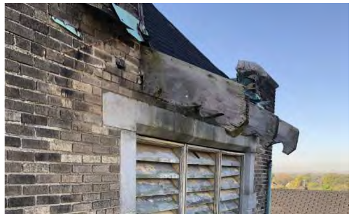
FIGURE A3.6 DIFFERENTIAL BRICK MOVEMENT UNDER EAVES; REMNANTS OF THE ORIGINAL STEPPED COPPER FLASHING; (NORTH ELEVATION)
