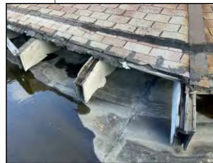
ROTTEN AND DAMAGED SHEATHING AT BRACKETS AT LOWER OVERHANG
