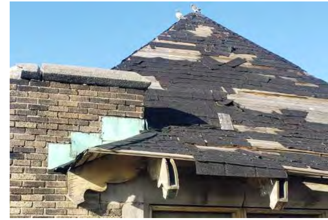
FIGURE A3.7 HIP ROOF IS IN VERY POOR CONDITION; WEATHERED AND DECAYED WOOD DECKING, MISSING/FALLEN SHINGLES AND EXPOSED DECKING AND ORIGINAL STEPPED COPPER FLASHING (EAST ELEVATION)
