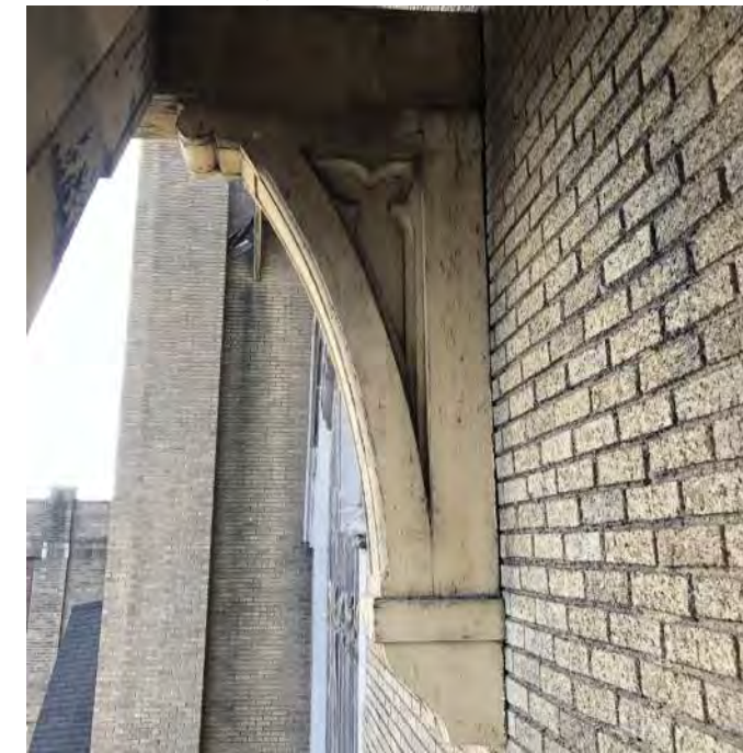
FIGURE A4.15 UNDERSIDE OF THE EAVES; PAINTED WOODEN BRACKET EAVE SUPPORT; (EACH BRACKET SHOULD BE INDIVIDUALLY EVALUATED)
