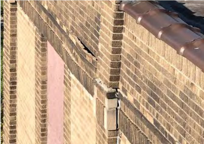
FIGURE A1.22 "ROLLING" BRICK DISPLACEMENT AT THE EXTERIOR PARAPET; BUCKLING AT PIER COLUMN
