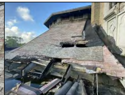
LOWER SLOPING ROOF AREA IN POOR CONDITION WITH DAMAGED SHEATHING AND SUPPORT RAFTERS
