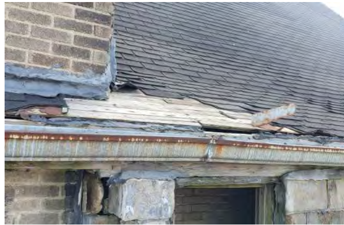
FIGURE A4.9 WEATHERED FASCIA BOARD; DECAYED WOOD DECKING; CURLED, FRAYED AND MISSING ASPHALT SHINGLES ABOVE ROOFTOP STAIR ENTRY.
