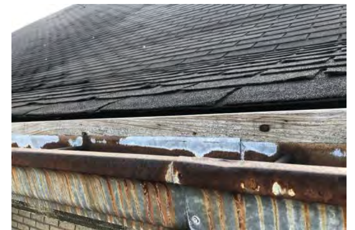
FIGURE A4.5 RUSTED GUTTER, CURLLED AND FRAYED ASPHALT SHINGLES
