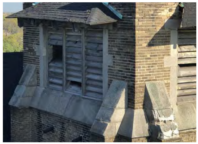
FIGURE A3.12 SOUTH WEST ELEVATION OF BELL TOWER; CRUMBLING STONE AT THE COLUMN CAP; BRICK MOVEMENT DIRECTLY UNDER THE ROOF
