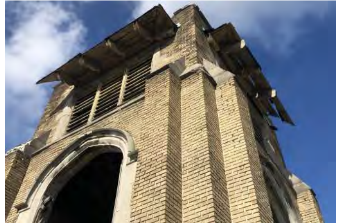
FIGURE A3.2 THE EAVE OVERHANG SHOWS EXTENSIVE WOOD DECAY AND DETERIORATION
