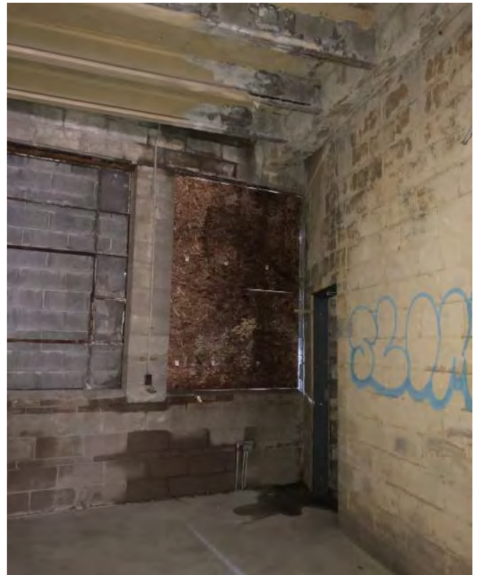
FIGURE INT 1.11 BOARDED UP FORMER WINDOW OPENINGS
