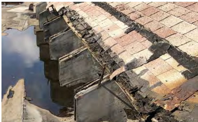
FIGURE A2.13 DECORATIVE WOOD EAVE SHOW SIGNS OF DECAY AND ROT; SIGNIFICANT DETERIORATION OF THE ROOF PERIMETER EDGE; WITH POOLS OF WATER GATHERING UNDER THE EAVES
