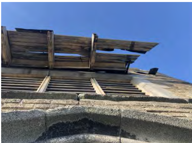
FIGURE A3.9 UNDERSIDE OF THE PAINTED DECORATIVE OVERHANGS; WEATHERED DETERIORATED WOOD DECKING (EAST ELEVATION)
