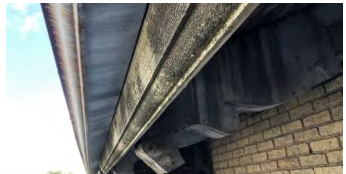
FIGURE A4.4 WEATHERED FASCIA BOARD WITH ATTACHED METAL GUTTER
