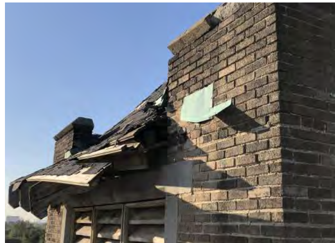
FIGURE A3.4 DECORATIVE WOOD OVERHANGS COLLAPSING AND OPEN AT ENDS TO INTERIOR; BRICK MASONRY SHOWS SIGNS OF DIFFERENTIAL MOVEMENT; REMAINING STEPPED COPPER FLASHING (EAST ELEVATION)
