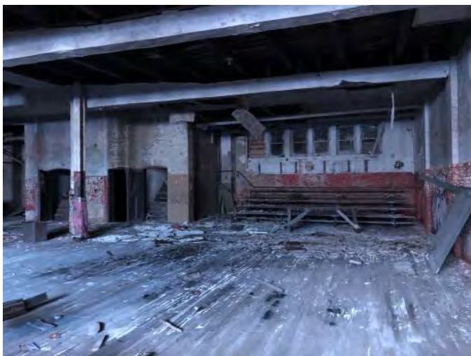
FIGURE INT.7 FAILED FINISHES AND DEBRIS IN LOWER LEVEL SPACES
