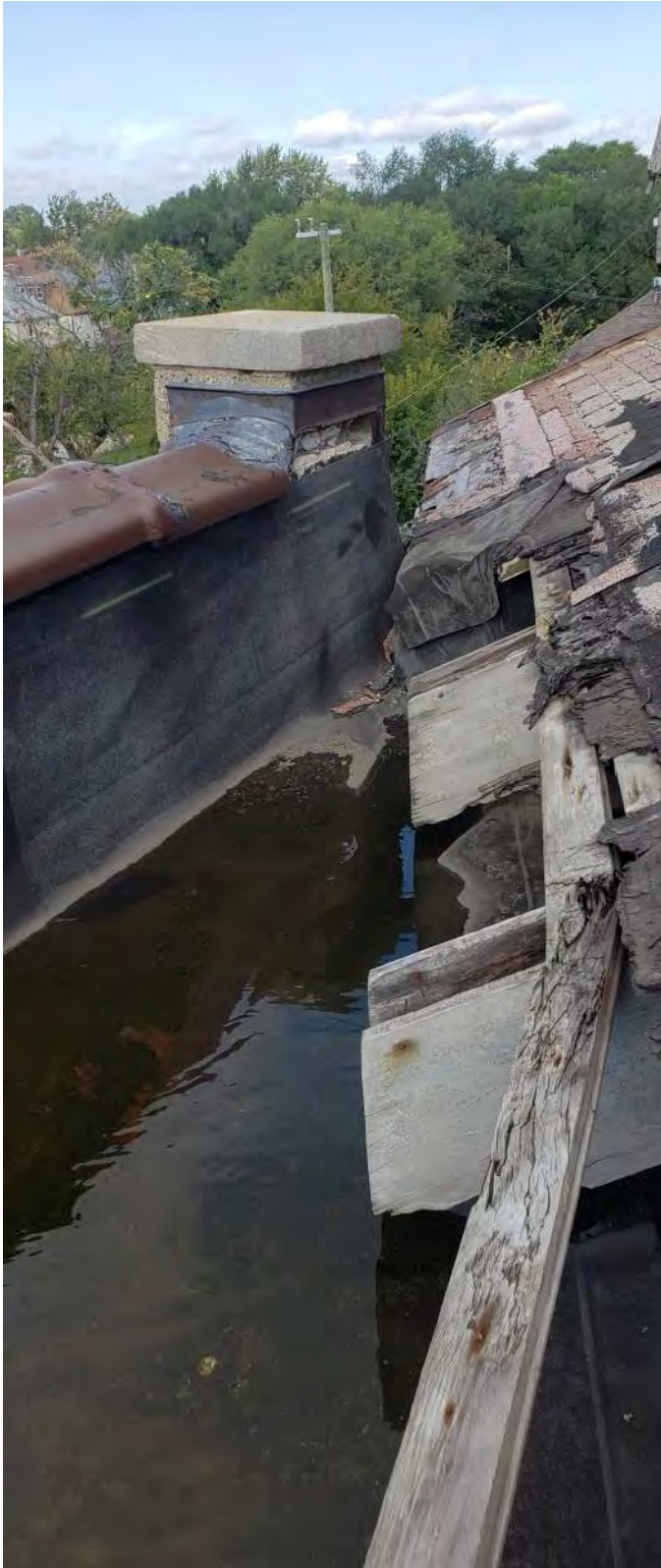
FIGURE A1.15 DETERIORATING CORNER COLUMN, UNFLASHSED MASONRY AT PIER COLUMN; 3" OR MORE PONDING WATER AT SOUTHWEST CORNER
