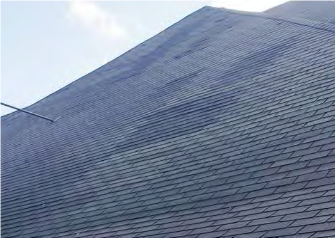
FIGURE A4.6 OVERVIEW OF NORTHERN ROOF; CURLLED, DISCOLORED, AND FRAYED ASPHALT SHINGLES; SHOW SIGNS OF DEPRESSIONS AND UNEVEN SURFACES ALONG THE ROOF
