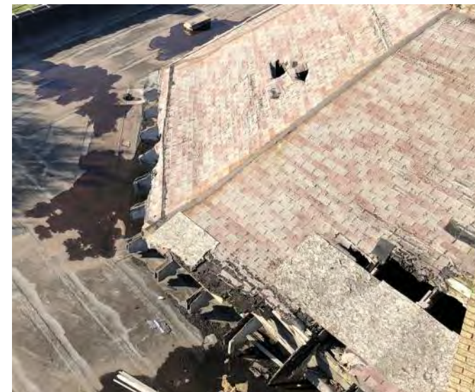
FIGURE A2.12 OVERVIEW OF THE HEPTAGON ROOF ABOVE, SHOWS THE EXTENT OF THE ROOF DETERIORATION WITH VARIOUS HOLES ALONG THE SURFACE
