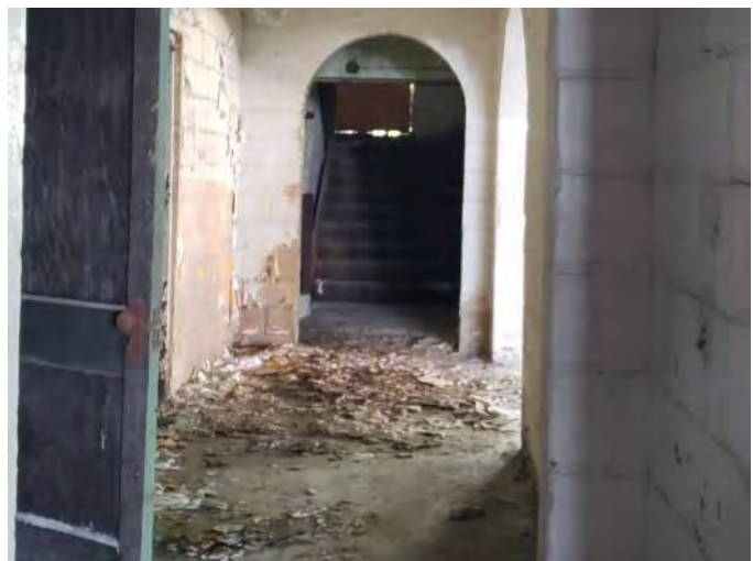
FIGURE INT.1.8 FAILED FINISHES AND DEBRIS IN ENTRYWAY AND CORRIDORS
