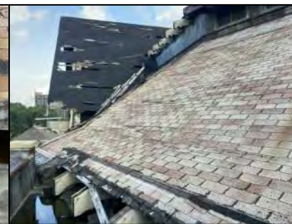
ROTTEN AND DAMAGED SHEATHING AND BRACKETS AT LOWER AND UPPER OVERHANGS
