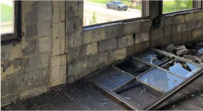
FIGURE INT 1.1 FALLEN OR MISSING WINDOWS; DETERIORATED MASONRY WALLS AND DEBRIS
