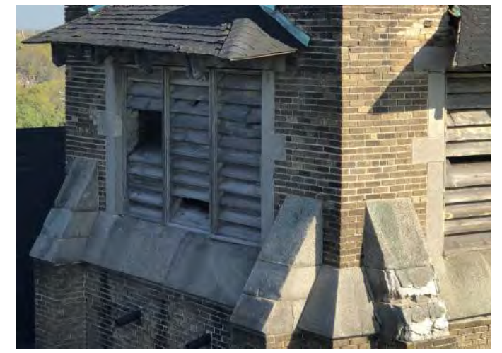
FIGURE A3.12 SOUTH WEST ELEVATION OF BELL TOWER; CRUMBLING STONE AT THE COLUMN CAP; BRICK MOVEMENT DIRECTLY UNDER THE ROOF
