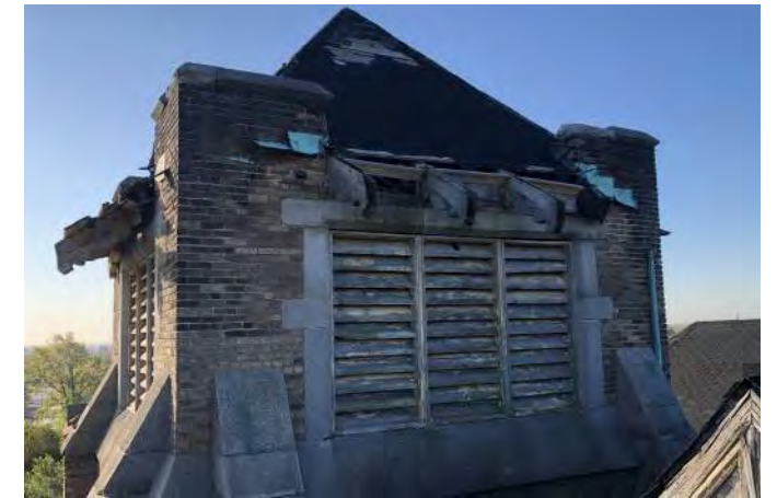
FIGURE A3.10 OVERVIEW OF THE BELL TOWER'S ROOF AND DECKING; THE DECKING ON TOP OF THE DECORATIVE EAVE HAS COMPLETELY DECAYED AND DETACHED FROM THE ROOF ASSEMBLY (NORTH ELEVATION)
