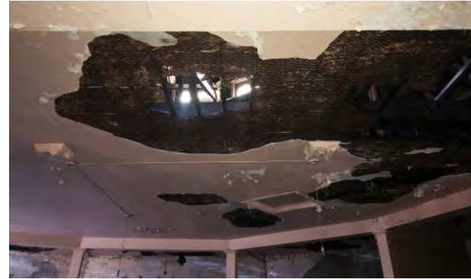
FIGURE A2.14 DETERIORATING INTERIOR PLASTER BELOW THE HEPTAGONAL ROOF STRUCTURE; SUN LIGHT IS VISIBLE THROUGH THE HOLE IN THE ROOF ABOVE
