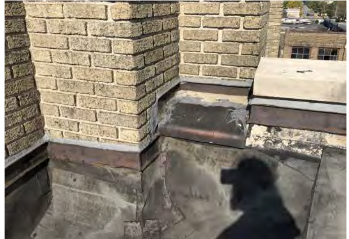
FIGURE A1.12 RUSTED FLASHING; WEATHERED SEALANTS, FLASHING MISSING AT THE UNDERSIDE OF THE COLUMN CAP
