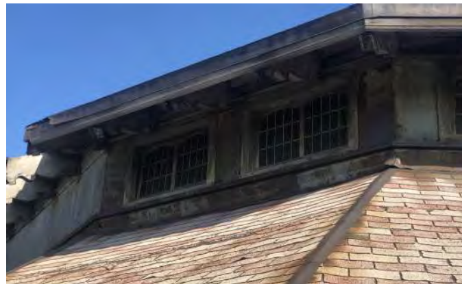
FIGURE A2.11 THE UPPER TIER OF THE POLYGONAL ROOF; VISIBLE RUST ON THE METAL WINDOW FRAMING AND ROOF HIP; METAL FLASHING IS CORRODING AND DETACHING FROM THE FASCIA BOARD AND HEAD OF LOWER ROOF
