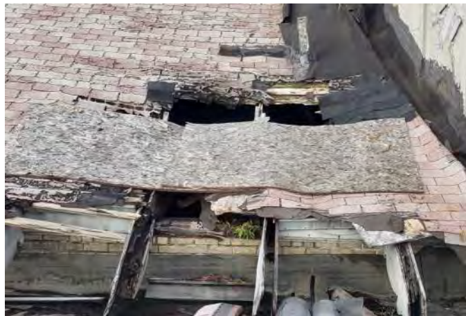
FIGURE A2.7 COMPLETE DETERIORATION AND DECAY OF THE DECORATIVE WOOD EAVES AND DECORATIVE RAFTER TAILS; THE LEVEL OF DETERIORATION MAY REQUIRE LOCALIZED REPAIRS TO ADJACENT ELEMENTS SUCH AS THE BRICK WALL BELOW
