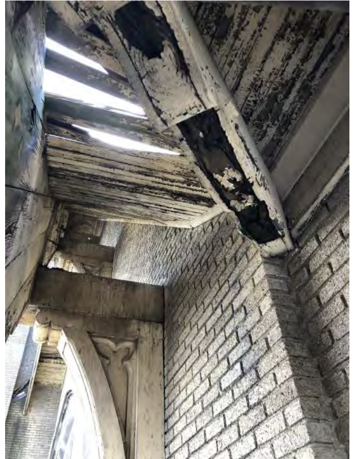
FIGURE A4.16 UNDERSIDE OF EAVES ON THE EAST ELEVATION AT THE MAIN ENTRANCE; WOOD DECKING IS DETERIORATION AT THE EAVE; MISSING WOOD DECKING; WEATHERED AND DECAYING SUPPORT BRACKETS
