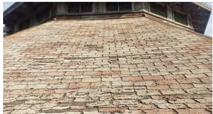
FIGURE A2.2 SURFACE DEPRESSIONS ALONG THE ROOF; CURLLED, DISCOLORED AND FRAYED ASPHALT SHINGLES; RUSTED METAL FLASHING UNDER THE UPPER WINDOWS
