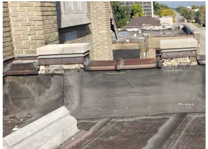
FIGURE A1.11 FLASHING MISSING UNDER COLUMN CAP
