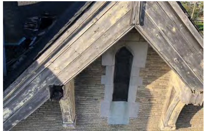
FIGURE A4.24 WEATHER AND FADED FASCIA BOARDS; DECAYED HOLLOWED WOODEN SUPPORT BRACKET
