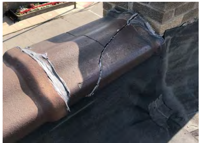
FIGURE A1.10 CRACKED CLAY TILES ALONG EAST ELEVATION
