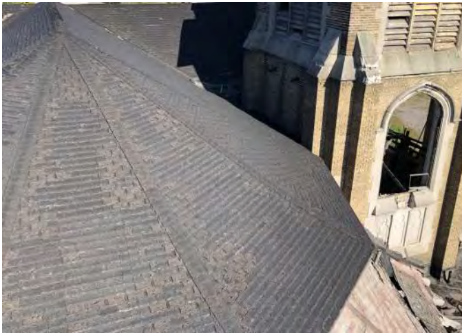
FIGURE A2.10 UPPER TIER OF HEPTAGON ROOF; WORN, MISSING CURLED, DISCOLORED, AND FRAYED ASPHALT SHINGLES
