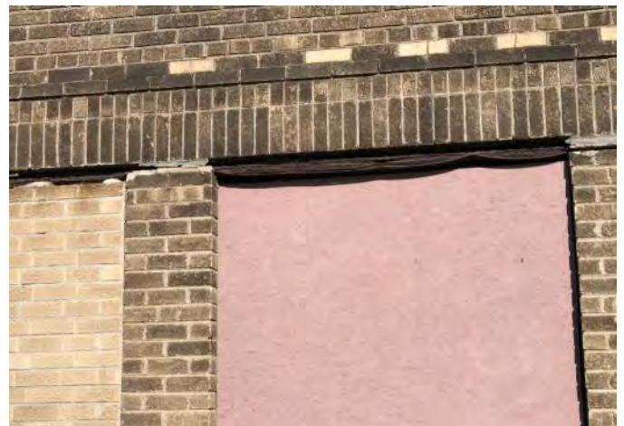
FIGURE A1.21 CORRODED AND EXPANDING STEEL LINTEL ABOVE THE WINDOWS ON THE THIRD FLOOR
