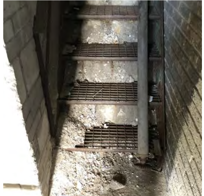
FIGURE INT 1.3 INTERIOR PLASTER HAS CRUMBLLED FROM THE WALLS, CEILING AND STRINGER BEHIND THE STAIR (LEADS TO THE ROOFTOP EXIT)
