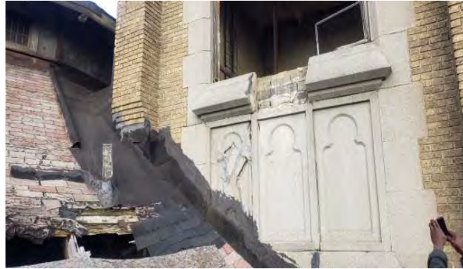
FIGURE A2.6 FAILURE OF THE FLASHING AT THE INTERSECTION WHERE THE POLYGONAL ROOF INTERSECTS WITH THE BELL TOWER; STAINING OF THE DECORATIVE STONE BY FLASHING SEALANT
