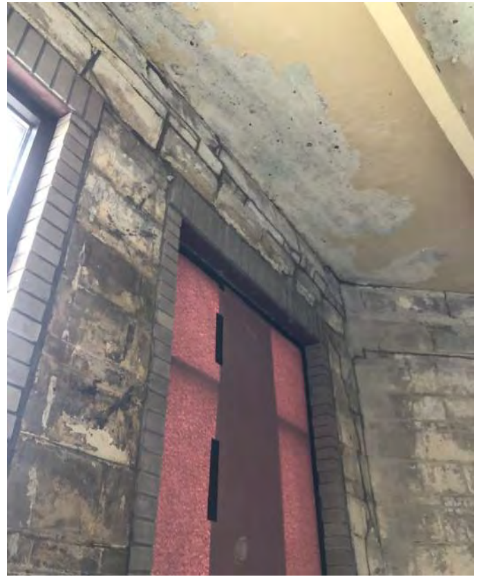
FIGURE INT 1.10 BUCKLING AND CRACKED MASONRY EXTERIOR WALLS
