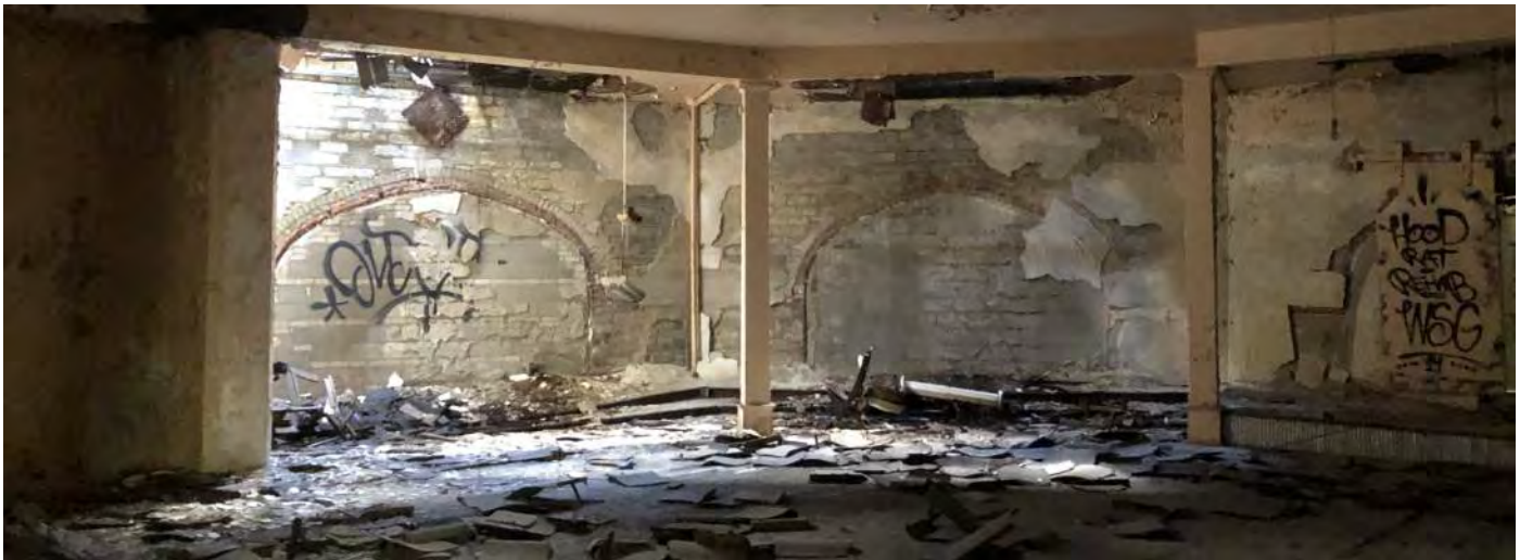
FIGURE INT.1.6 FAILED FINISHES AND DEBRIS IN CLASSROOMS OVER SANCTUARY; OPENINGS THRU ROOFS TO DAYLIGHT ABOVE
