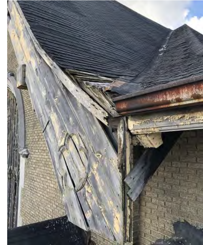
FIGURE 4.13 DECORATIVE FASCIA BOARDS ARE WEATHERED AND FADED; THEY ARE DETACHING FROM THE SUBSTRUCTURE. WOOD DECKING AT VALLEY TERMINATION IS EXPOSED, DECAYED WITH MISSING SHINGLES
