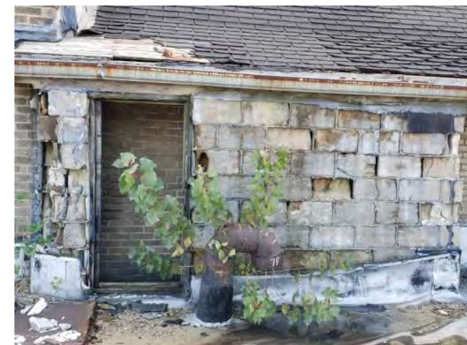
FIGURE A4.23 EXTENSIVE EXTERIOR MASONRY DETERIORATION AT ROOFTOP STAIR ENTRY/EXIT; MISSING AND DETERIORATED MORTAR JOINTS; DETACHED ROOFTOP STAIR ENTRY DOOR; DAMAGED DOOR FRAMING. DETACHED FLASHING AT THE UPTURN OF THE NORTH MEMBRANE ROOFING
