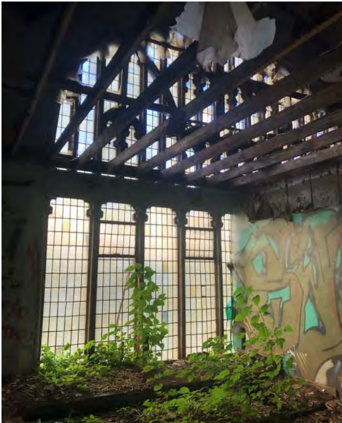
FIGURE INT 1.8 FAILED FINISHES AND VEGETATION IN SANCTUARY MEZZANINE OPEN TO THE ELEMENTS ABOVE
