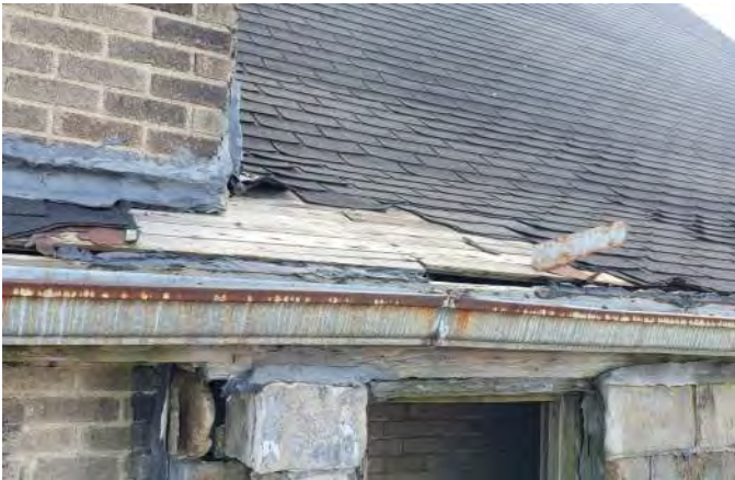
FIGURE A4.9 WEATHERED FASCIA BOARD; DECAYED WOOD DECKING; CURLLED, FRAYED AND MISSING ASPHALT SHINGLES ABOVE ROOFTOP STAIR ENTRY.
