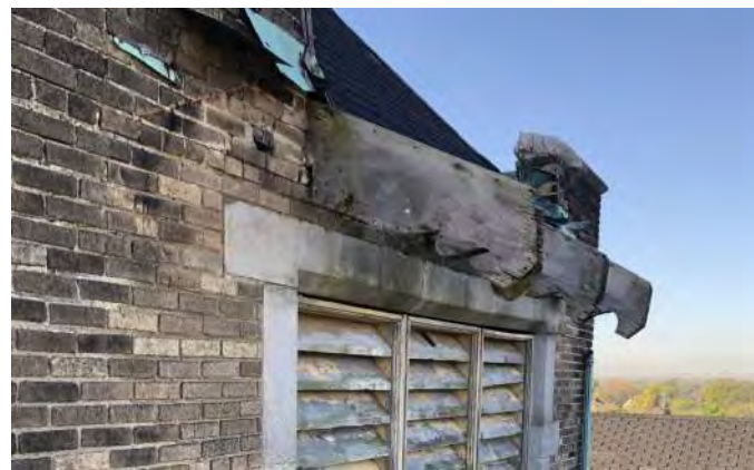
FIGURE A3.6 DIFFERENTIAL BRICK MOVEMENT UNDER EAVES; REMNANTS OF THE ORIGINAL STEPPED COPPER FLASHING; (NORTH ELEVATION)
