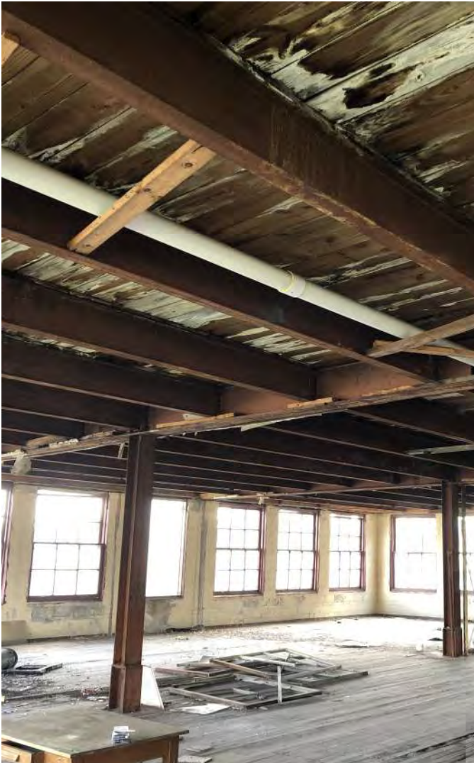
FIGURE INT 1.2 WATER STAINED AND LOOSE WOOD DECKING; OXIDIZED STRUCTURAL BEAM AND COLUMNS; VARIOUS DEBRIS; AT 1917 ADDITION INTERIORS
