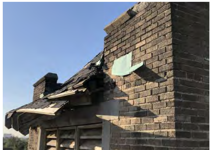
FIGURE A3.4 DECORATIVE WOOD OVERHANGS COLLAPSING AND OPEN AT ENDS TO INTERIOR; BRICK MASONRY SHOWS SIGNS OF DIFFERENTIAL MOVEMENT; REMAINING STEPPED COPPER FLASHING (EAST ELEVATION)
