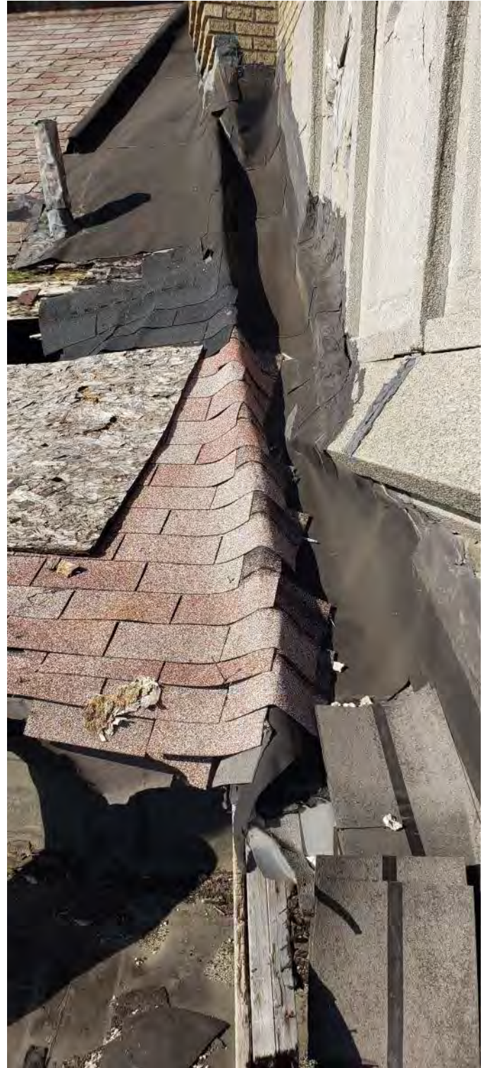
FIGURE A2.13 IMPROPER FLASHING AND PATCHING AT THE VALLEY JUNCTION BETWEEN THE POLYGONAL ROOF AND BELL TOWER; THE ASPHALT SHINGLES ARE NOT PROPERLY TERMINATED; EXCESSIVE USE OF ROOFING MASTIC ALONG THE BELL TOWER WALL; DETERIORATED ROOF VENT NEAR THE LARGE HOLE IN THE ROOF.
