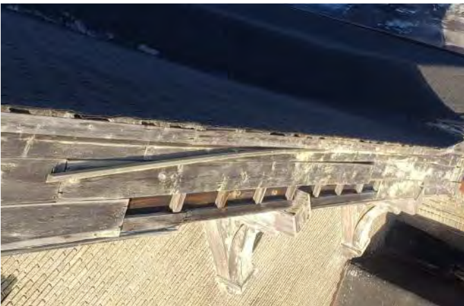
FIGURE A4.14 MISSING WOOD FASCIA BOARDS AT EAST ELEVATION
