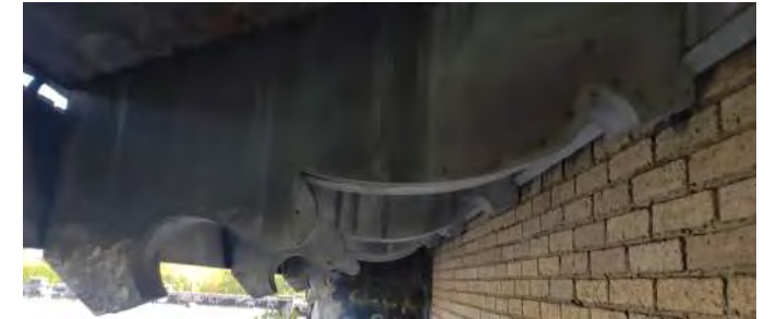
FIGURE 4.2 DECORATIVE WOOD EAVE, SIDE ELEVATION APPROX. LENGTH 3'-4"; IN FAIR CONDITION
