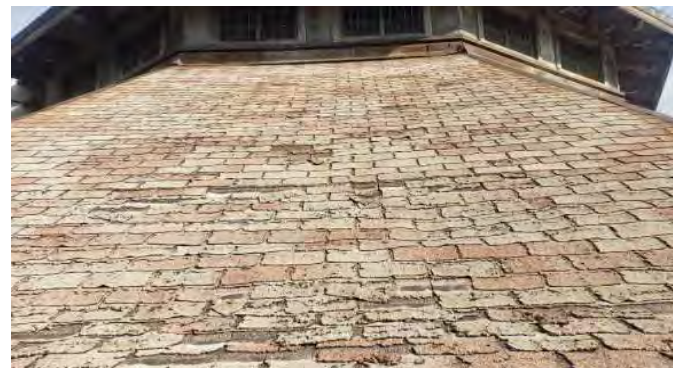
FIGURE A2.2 SURFACE DEPRESSIONS ALONG THE ROOF; CURLED, DISCOLORED AND FRAYED ASPHALT SHINGLES; RUSTED METAL FLASHING UNDER THE UPPER WINDOWS
