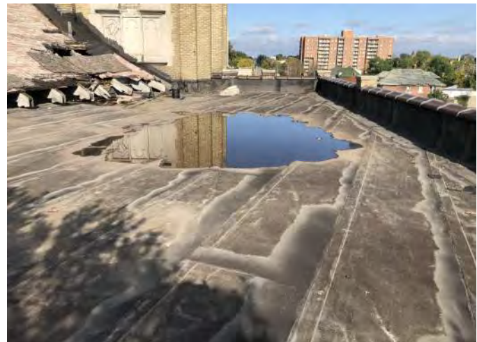
FIGURE A1.2 OVERVIEW LOOKING NORTH AT THE FLAT ROOF WITH STANDING WATER; FRAYED RUBBER ROOF SEAMS; PARAPET FLASHING
