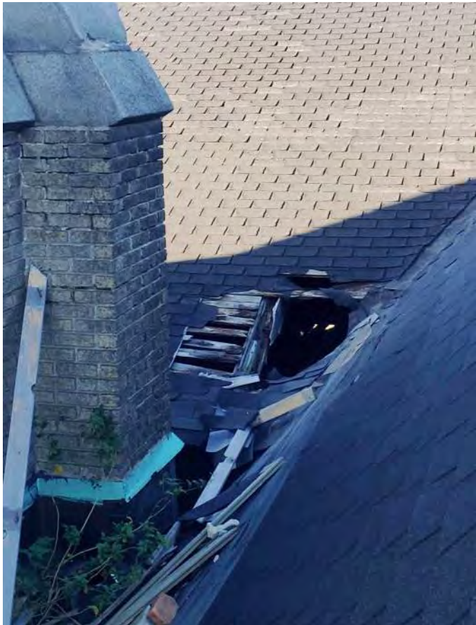
FIGURE A4.17 LARGE HOLE IN THE ROOF; DETERIORATED SHINGLES, WOOD DECKING AT THE ROOF VALLEY ; FALLEN WOOD DECKING FROM THE BELL TOWER ROOF ABOVE
