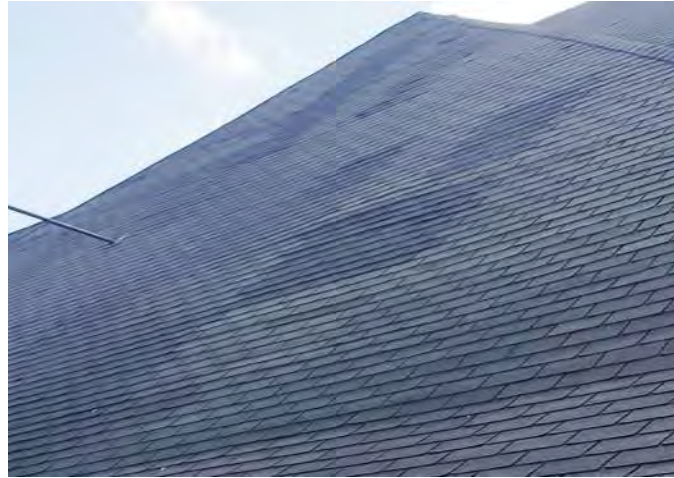
FIGURE A4.6 OVERVIEW OF NORTHERN ROOF; CURLED, DISCOLORED, AND FRAYED ASPHALT SHINGLES; SHOW SIGNS OF DEPRESSIONS AND UNEVEN SURFACES ALONG THE ROOF
