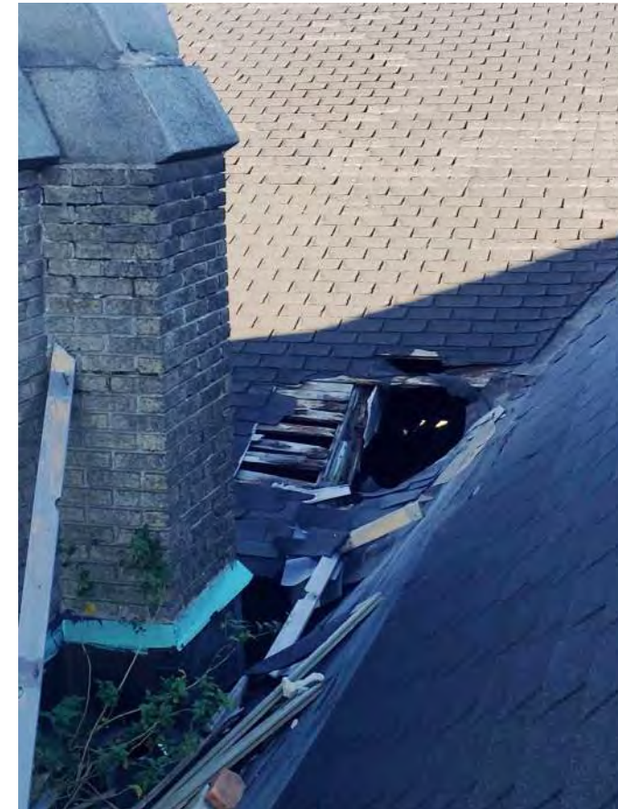
FIGURE A4.17 LARGE HOLE IN THE ROOF; DETERIORATED SHINGLES, WOOD DECKING AT THE ROOF VALLEY; FALLEN WOOD DECKING FROM THE BELL TOWER ROOF ABOVE
