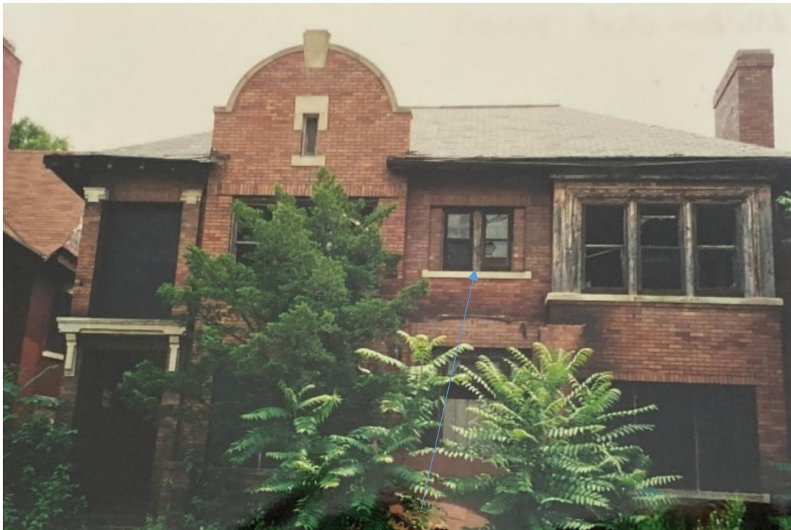
Photo taken in 2000. COA required that new windows match designation slide conditions
