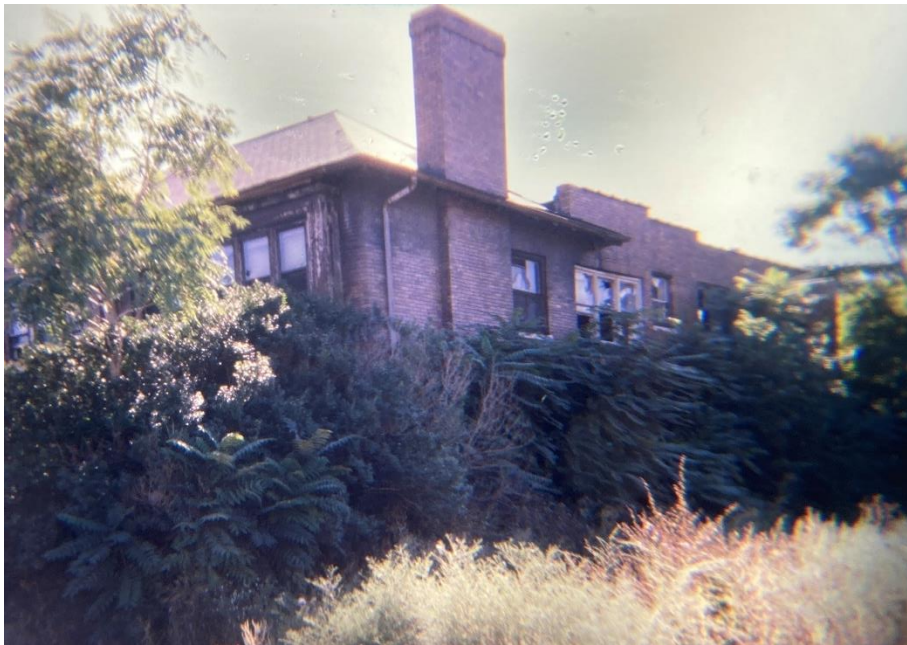
Designation slides, taken in 1980. Note the level of deterioration at the building's windows
