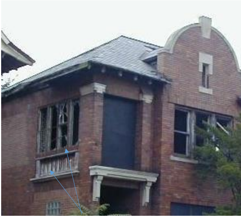
Condition in 2000. Note that this location included 4, double-hung, mullioned windows within this opening. There is a brick sill with an opening below that is infilled with wood paneling. Also, note location of historic/original stone sill
