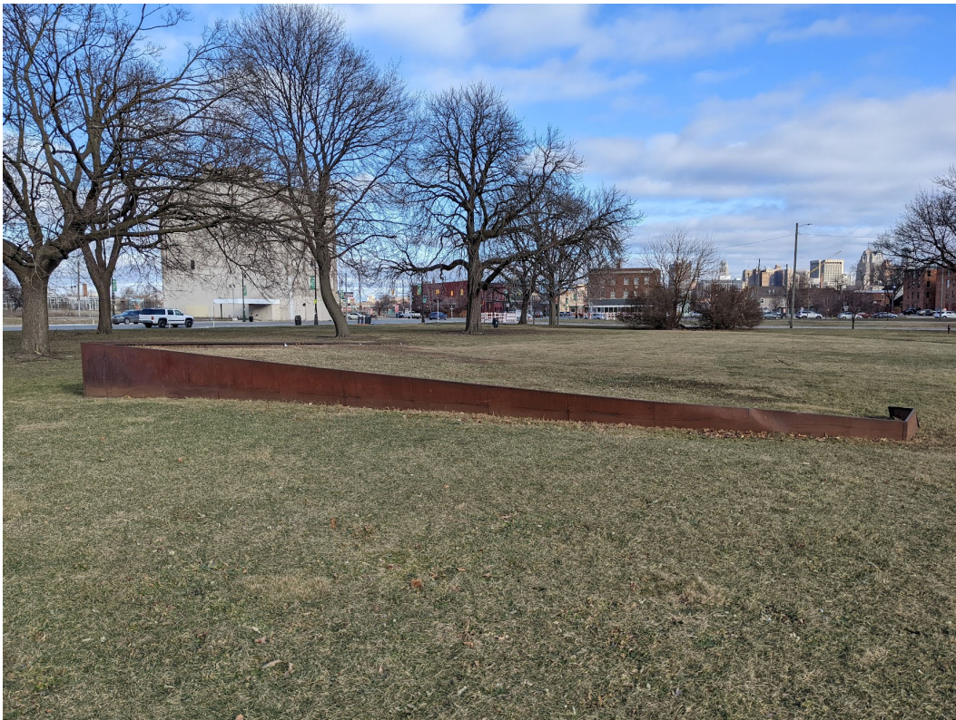
Steel retaining wall in park, west of the axial drive. Staff photo, January 14, 2022.
