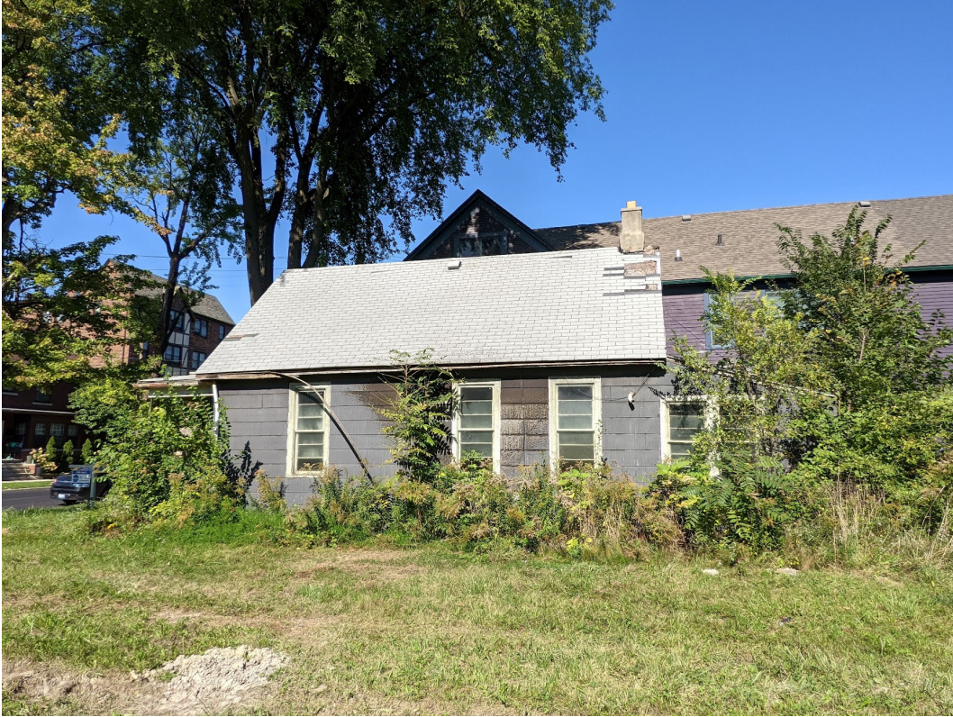
Side view (south elevation) of 1532 Van Dyke, looking north. Note original wood windows of eccentric design.
