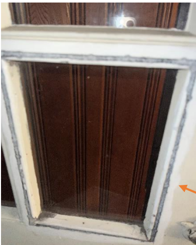
Mold growing around window pane that was replaced
