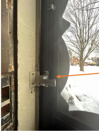
Screen door doesn't lock
