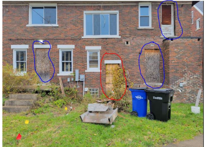
Site photo 4, by Applicant: (Southeast) rear elevation indicating location of basement door proposed to be bricked in (red) and doors to be replaced (blue).
