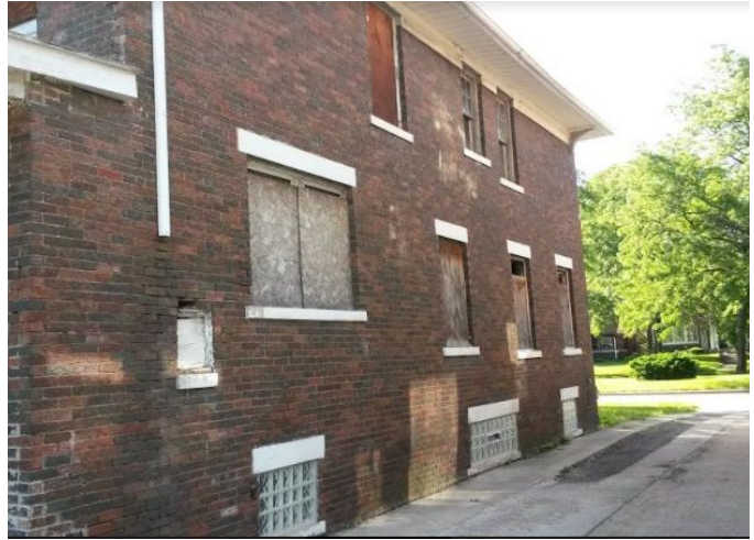
Site Photo 5, by Applicant, November 2014: (Northeast) side elevation showing applicant's stated condition with soffits and windows before work done.
