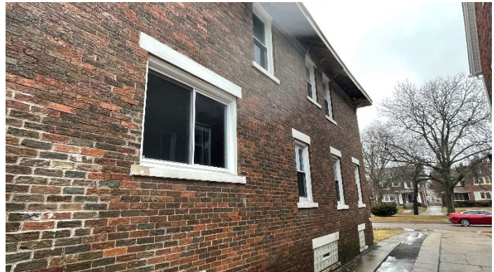
Site Photo 6, by Staff, February 17, 2022: (Northeast) side elevation showing soffits removed, original windows replaced with vinyl
