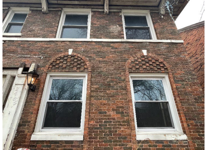
Site Photo 3, by Staff February 17, 2022: (Northwest) front elevation showing detail of front roof brackets, soffits and windows.
