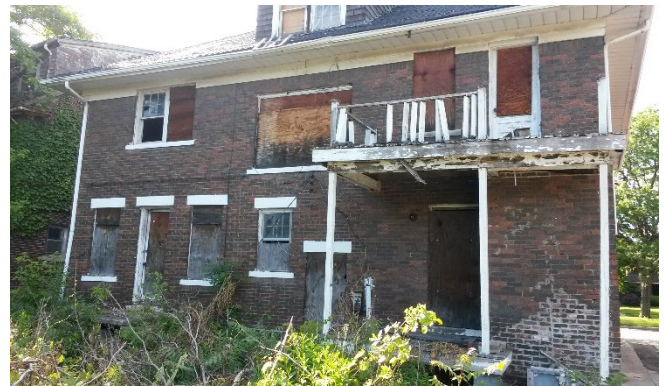
Site Photo2, by Applicant: (Southeast) rear elevation showing applicant's stated condition on Nov. 2014, with soffits and some windows in place.
