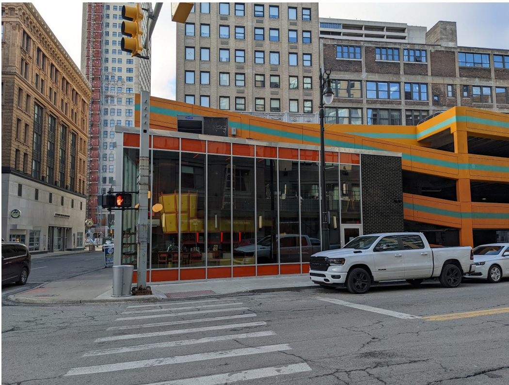
Current view towards the west of 1405 Griswold, at Grand River, showing work already completed. Griswold Street Elevation shown. Staff photo, January 14, 2022.
