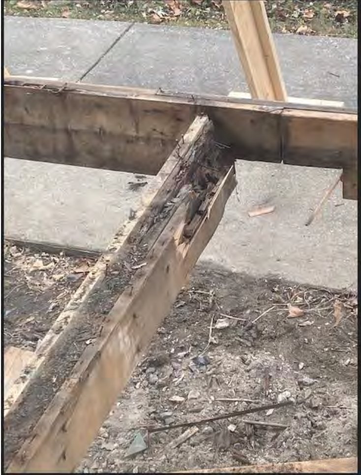
Condition of original porch: Rotten Wood / Missing Footing
