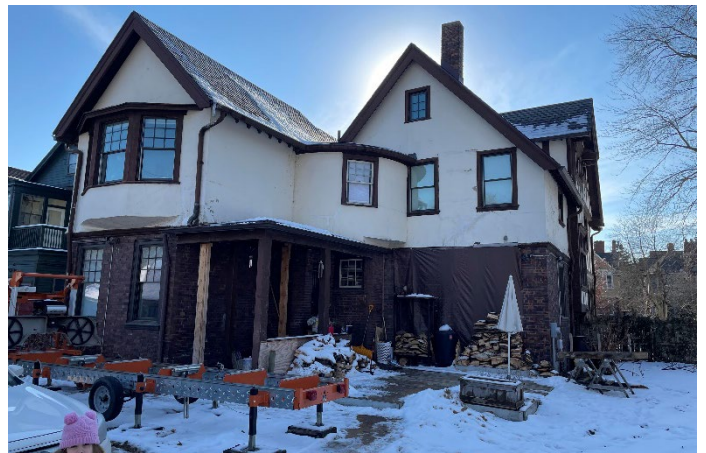
Site Photo 2, by applicant: (Northeast) rear elevation showing location of proposed addition.
