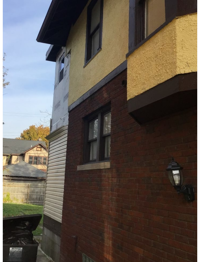
Site Photo 6, by applicant: (West) side elevation showing current condition by previous owner.
