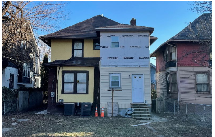
Site Photo 2, by Staff January 21, 2022: (Northwest) rear elevation showing reconstructed rear portion of the house.
