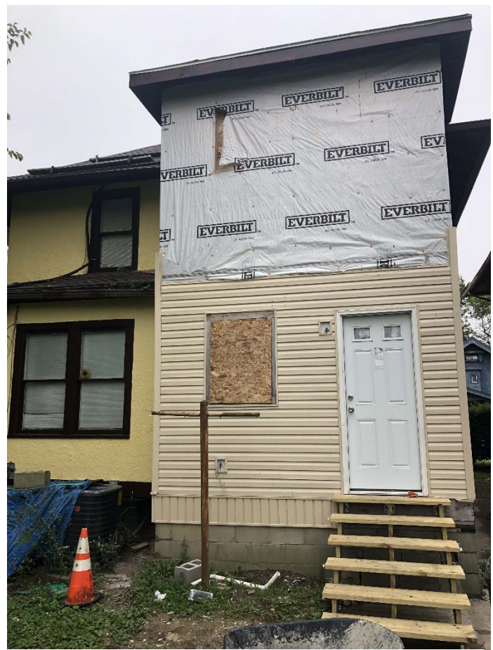
Site Photo 5, by applicant: (Northwest) rear elevation showing current condition as started by previous owner.
