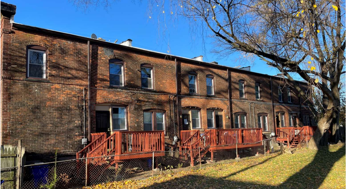
Site Photo 2, by Staff November 19, 2021: (Northeast) rear elevation showing installed vinyl windows on first and second floors.
