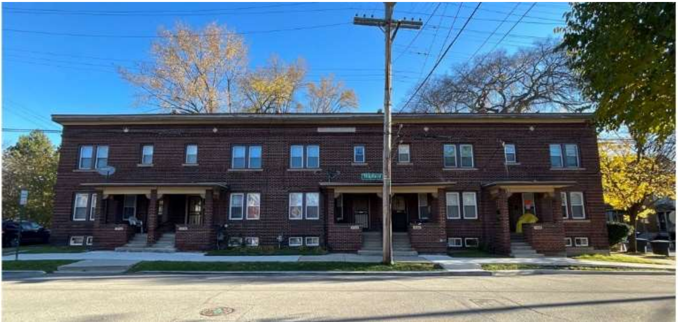
Site Photo 1, by Staff November 19, 2021: (Southwest) front elevation showing work complete of vinyl window installation and painted masonry on first floor window sills and capstones of the front porches. The BSEED stop work notice can be seen on the right-most entrance.
