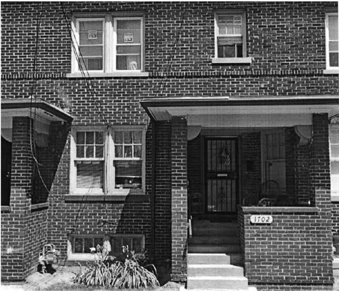
Site Photo 3, Google Streetview Aug. 2019: (Southwest) front elevation showing original 1 st , 2 nd and basement windows with newly installed vinyl windows in upper left.
