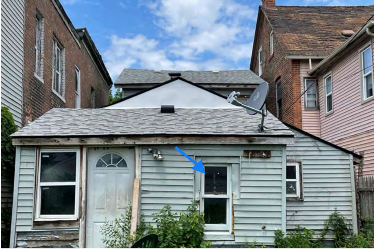
DETERIORATION TO EXISTING WINDOWS
