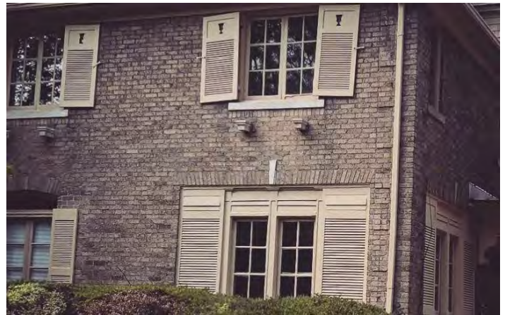
Site Photo7, close up of photo 3: (South) front elevation showing details of front elevation shutters and wood paneling.
