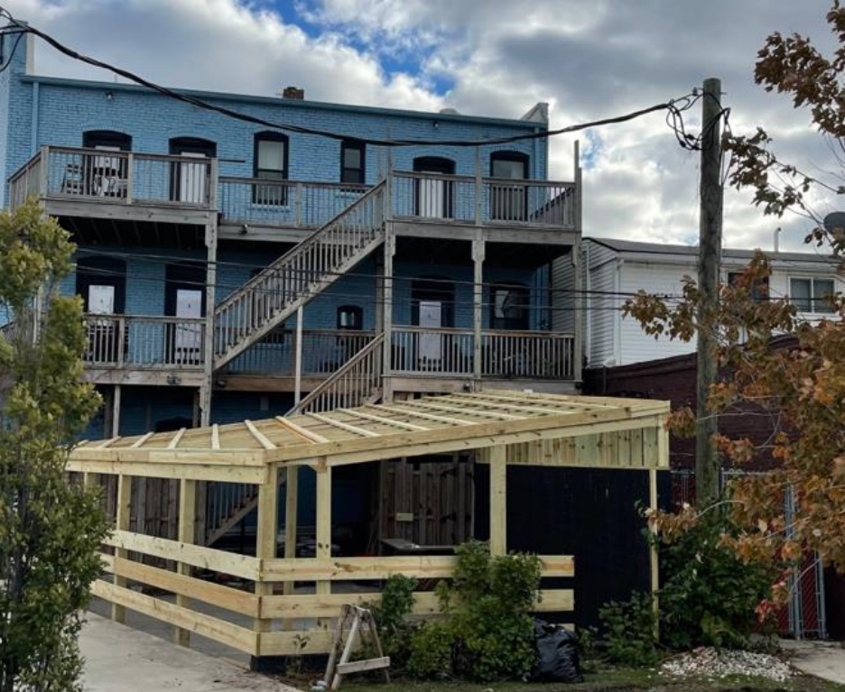
2104 Michigan, current appearance. Rear covered patio/trellis proposed for proposal. Note, that the work has been initiated without HDC approval
