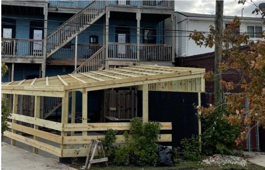
Current appearance. Covered patio area installed in October 2021 without HDC approval/COA
