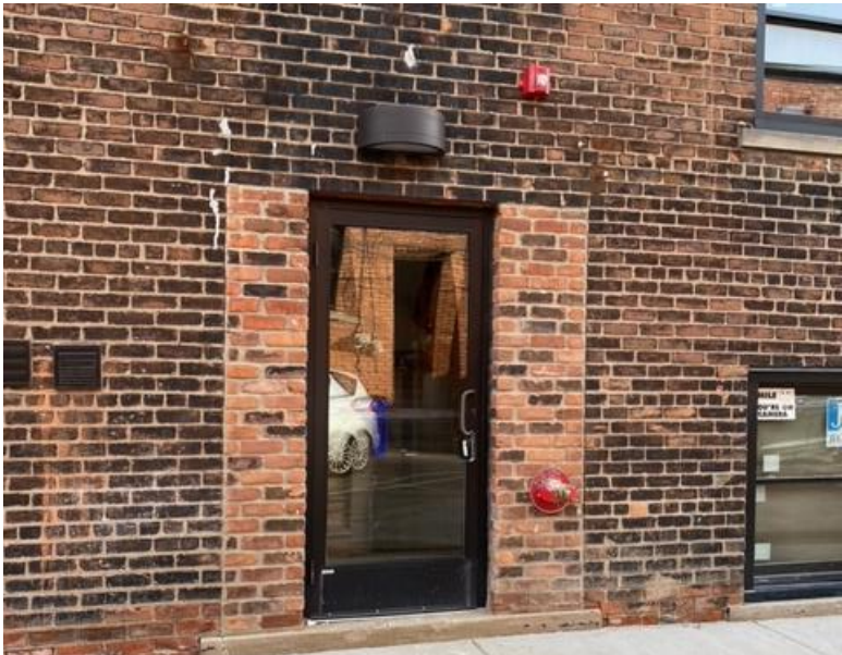
New aluminum door at west/side elevation. Replaced non-historic steel door. Brick infill was present in 2018.
