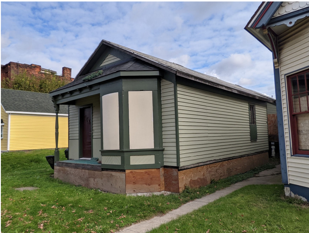
View of existing conditions at 2238 Wabash. The current skirt boards are temporary plywood enclosures. Staff photo, November 2, 2021.
