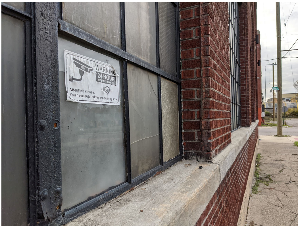
Detail view of steel sash windows and concrete sill/brick at first floor. Staff photo, November 2, 2021
