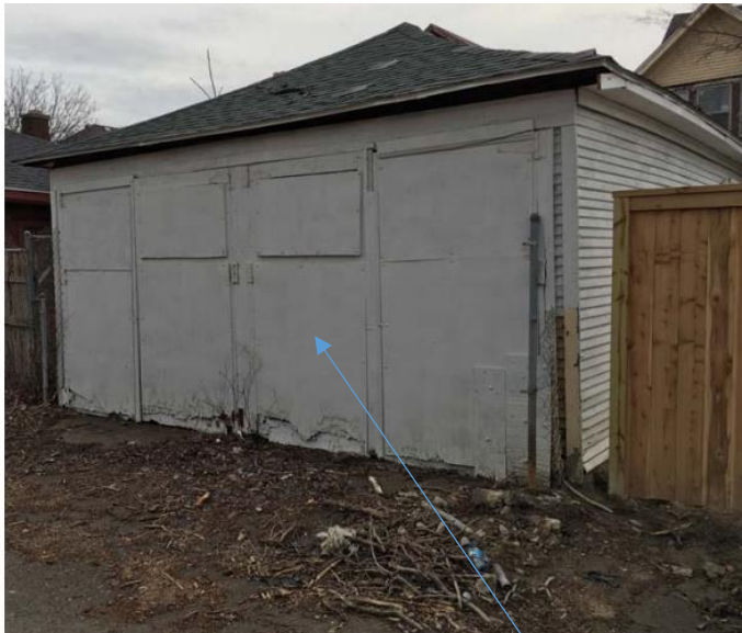
In 2017, the Commission approved the replacement of these door. Condition prior to the current work
