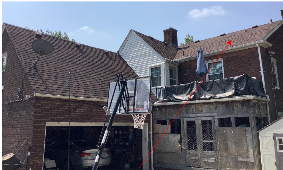
Rear elevation. Note the number of incompatible alterations to include the rear one-story enclosed porch, vinyl windows, and vinyl siding. The new panels represent an additional non-compatible element, in staff's opinion
