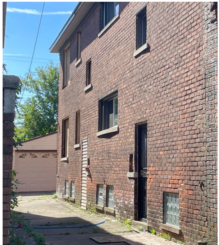
Site Photo 4, by Staff September 30, 2021: (East) rear side elevation showing door removed and replaced with vinyl siding, windows removed and replaced with plywood, basement windows replaced with glass block, and soffits covered in vinyl with metal fascia. New garage siding/doors in the background is not part of this application.
