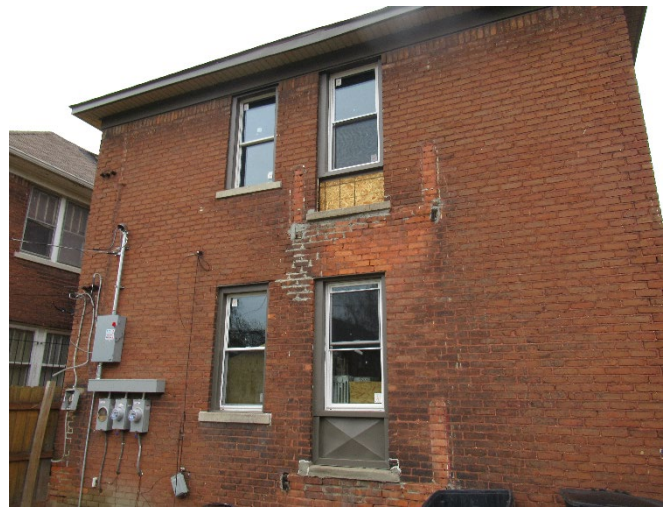
Site Photo 5 by Applicant showing vinyl soffit, metal fascia, removed rear porch/balconies, removed rear doors/windows and replaced with vinyl paneling and vinyl windows.
