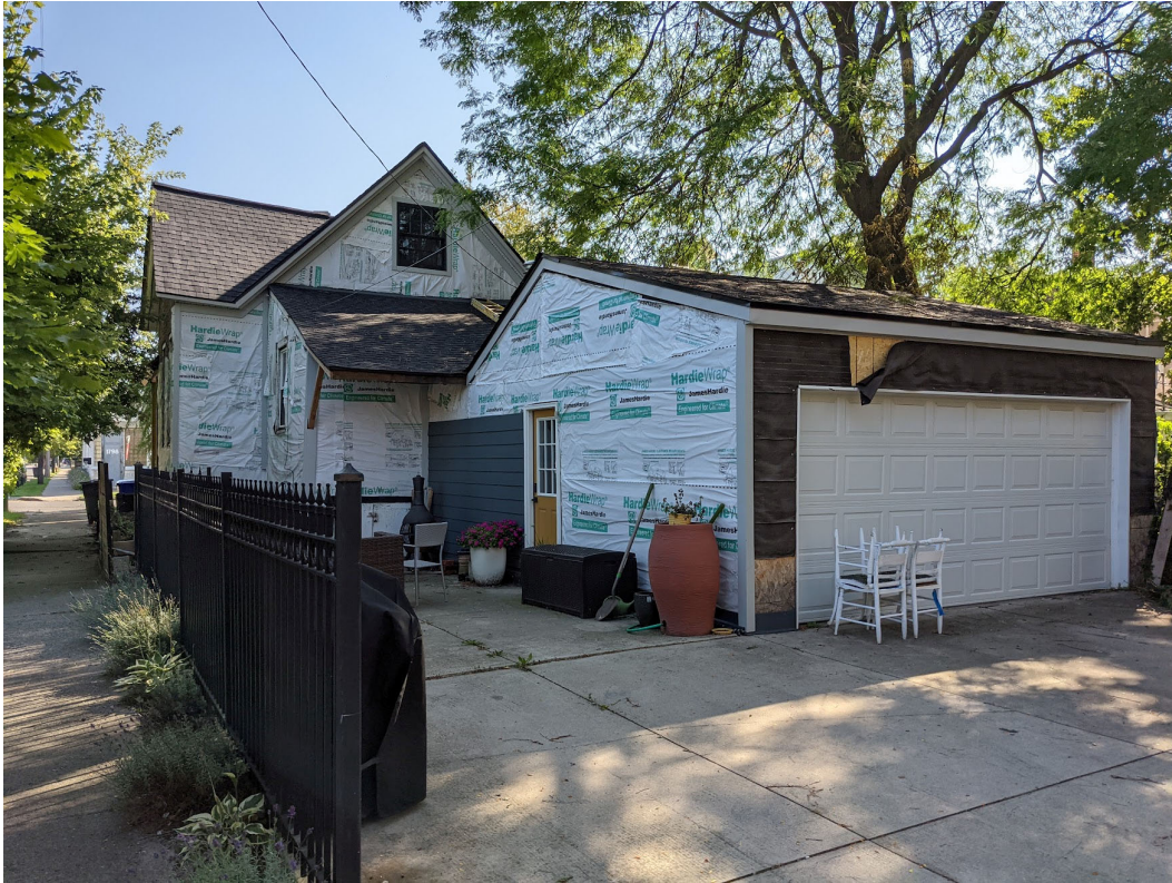
View of existing conditions at rear of 1801 Wabash, view to the east from Marantette. Staff photo, September 17, 2021.
