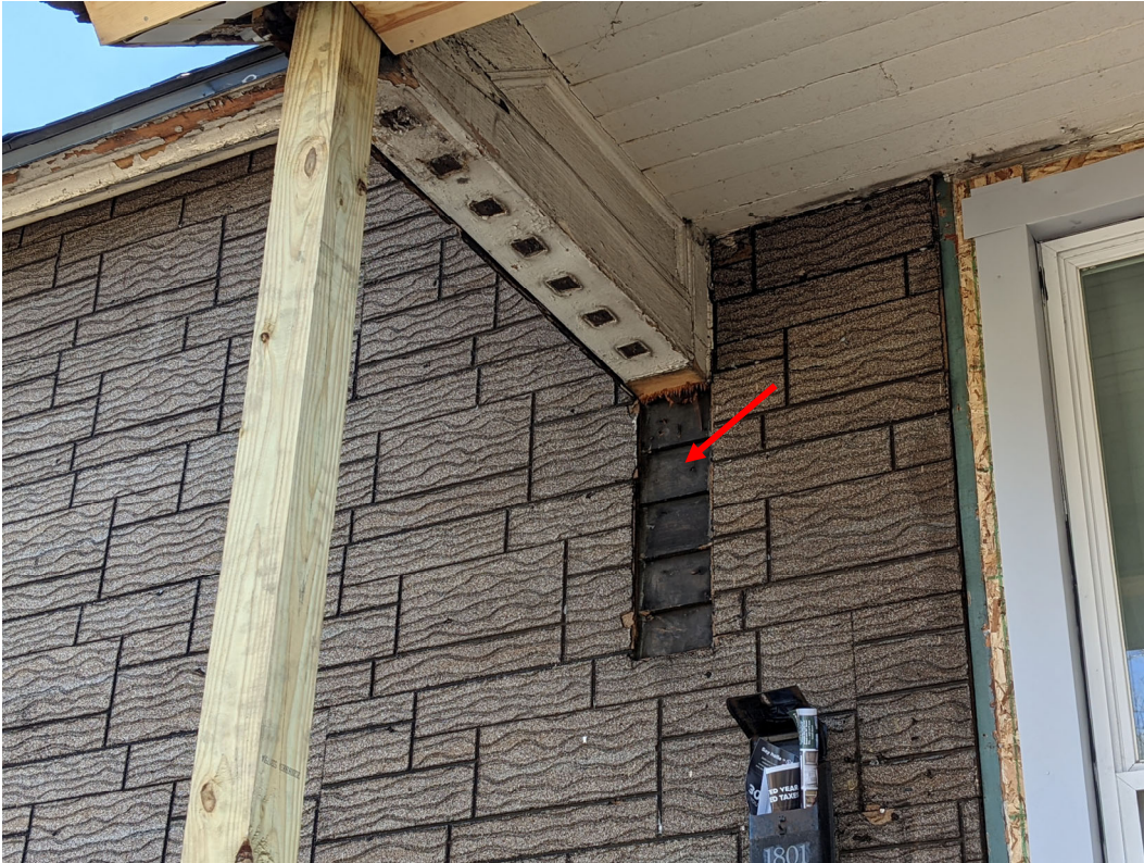
Detail view of porch along Marantette, showing new pressure-treated post and an evident area of original wood siding intact below the asphalt cladding. The siding is dirty with soot, and can likely be cleaned and painted. Staff photo, March 29, 2021.
