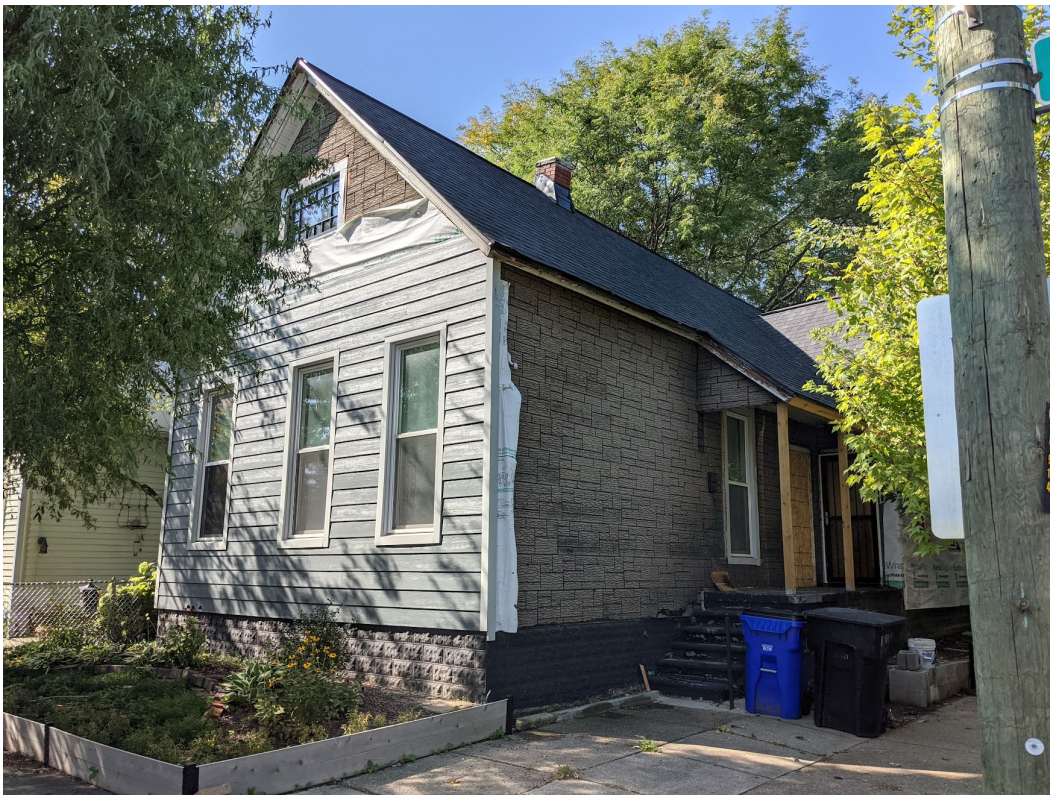
View of existing conditions at 1801 Wabash, view to the southwest. Staff photo, September 17, 2021.
