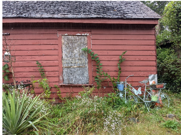
Site Photo 5, by Staff Sept. 21, 2021: (North Elevation, towards rear) Garage leaning east and sinking; note slope in windowsill.
