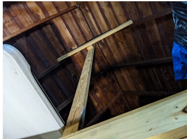
Site Photo 6, by Staff Sept. 21, 2021: (Garage ceiling) Applicant has previously attempted extensive bracing, under roof.
