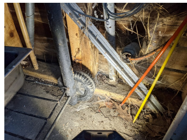
Site Photo 7, by Staff Sept. 21, 2021: (Garage wall) Applicant attempted bracing and repairs at studs/bottom plate, typical of several areas.
