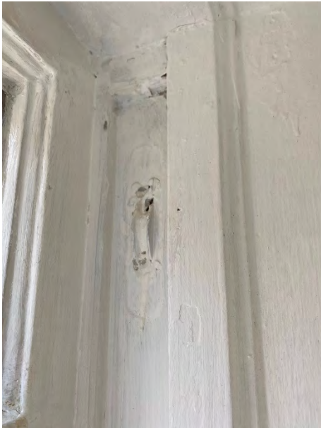
Operating hardware missing or inoperable
