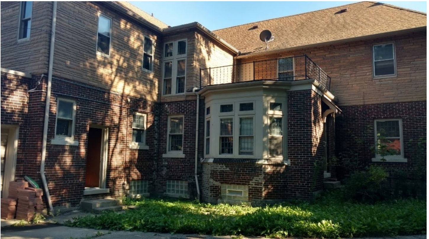
535 Arden Park. View of rear facade before windows were replaced and metal railing removed. Applicant photo.
