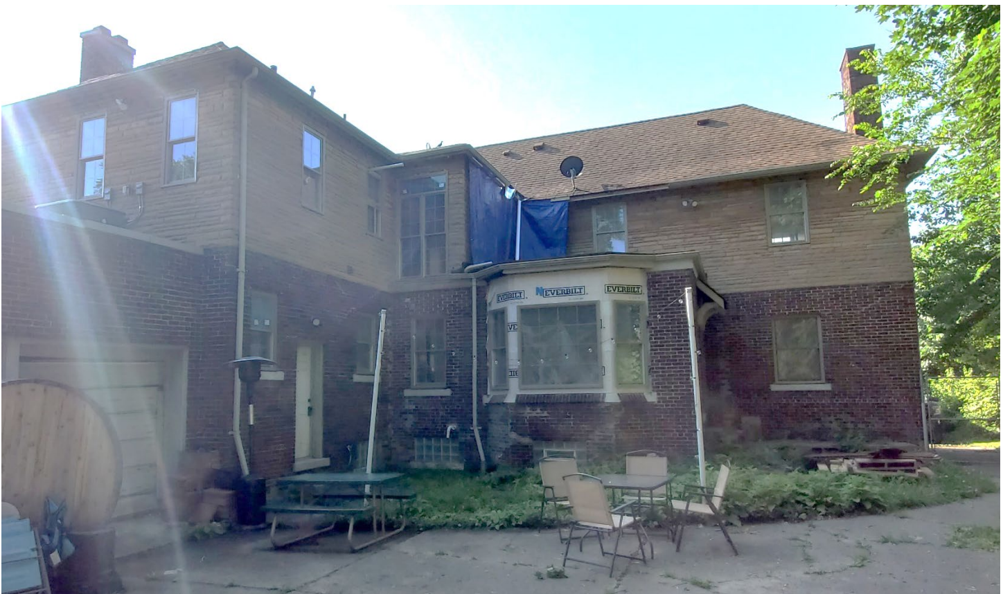
535 Arden Park. View of existing conditions at rear facade – windows replaced and metal railing removed without HDC approval. Applicant photo.
