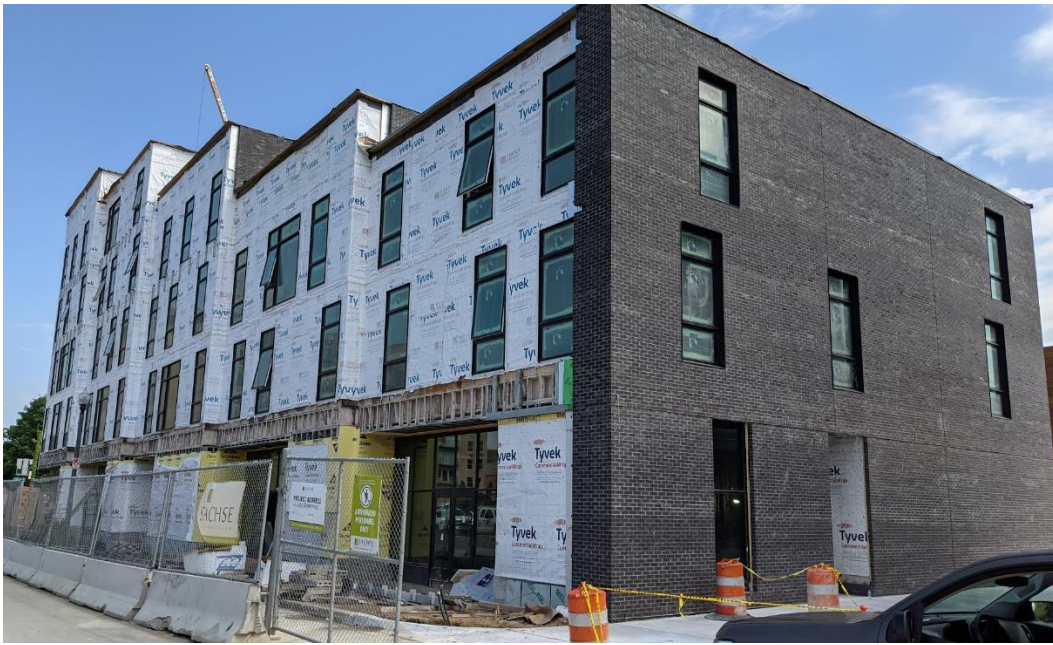
200 Edmund Place, current appearance from the southwest (alley elevation); staff photo, June 4, 2021.
