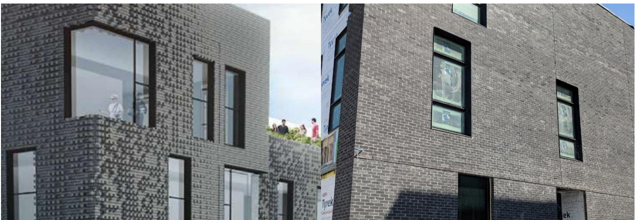
Original design from 2016 (left) versus current photo at the alley elevation (right) as constructed. It is not clear to staff if this is the effect meant to serve as “variegated” brick. The as-built appearance here (brick type “BR-1”, per the drawings) is plain and monolithic with almost no discernible variety or texture, whereas the approved brick effect is markedly textural, giving a robust, pixelated effect with strong shadows. Staff photo, 6/4/21.
