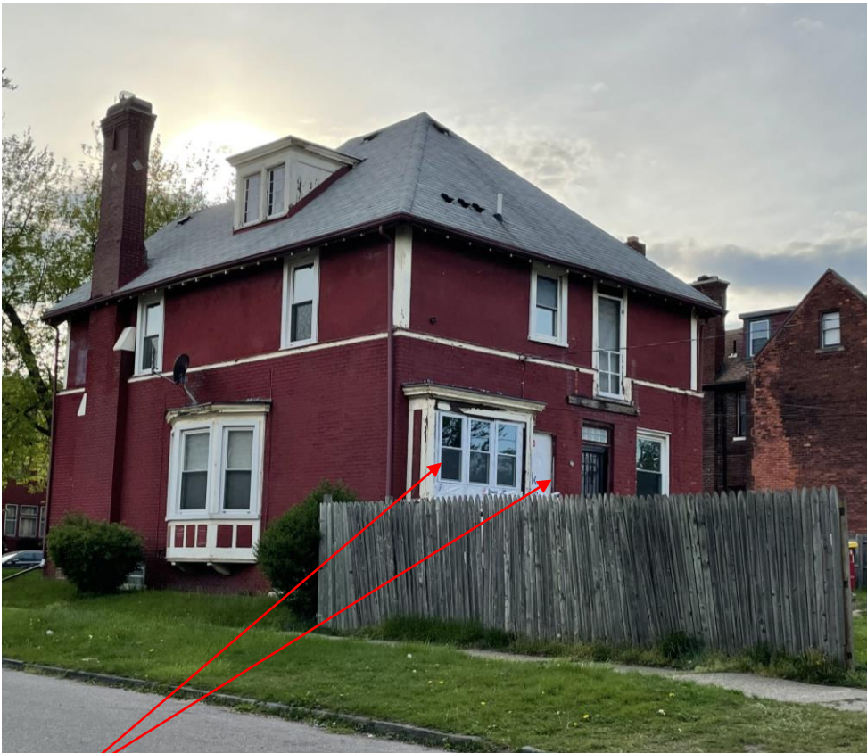
Rear elevation, current condition. Note that the three posed vinyl windows have been installed and the single rear window has been removed without HDC approval
