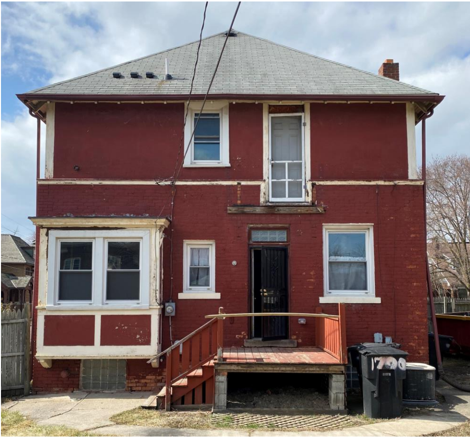
Rear elevation, PRIOR TO unapproved recent window removals
