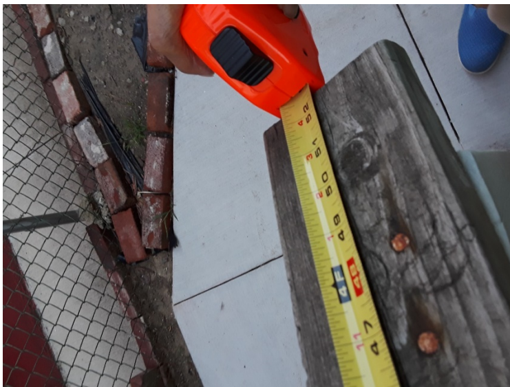
End of top rail for side porch is 52 ½ inches long. It will be replaced by a new wood rail.
