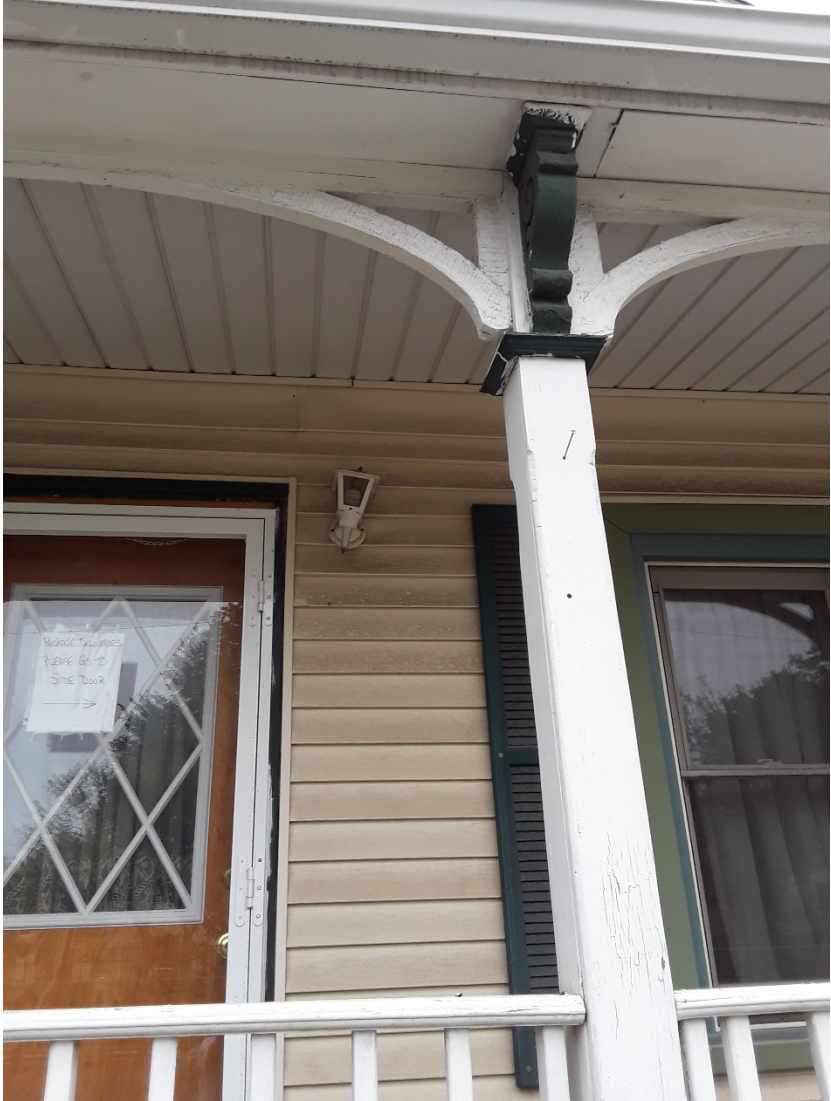
New porch light will be installed on both side of front door.
