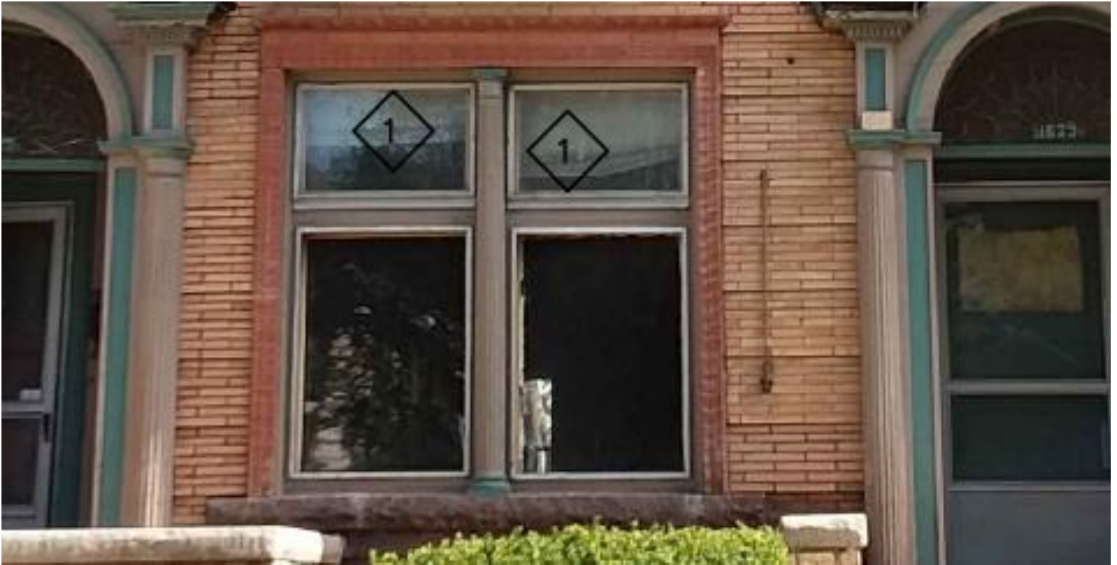
Front elevation window at first story, prior to unapproved work. Note, pilaster, wood trim, fixed windows and fixed transom
