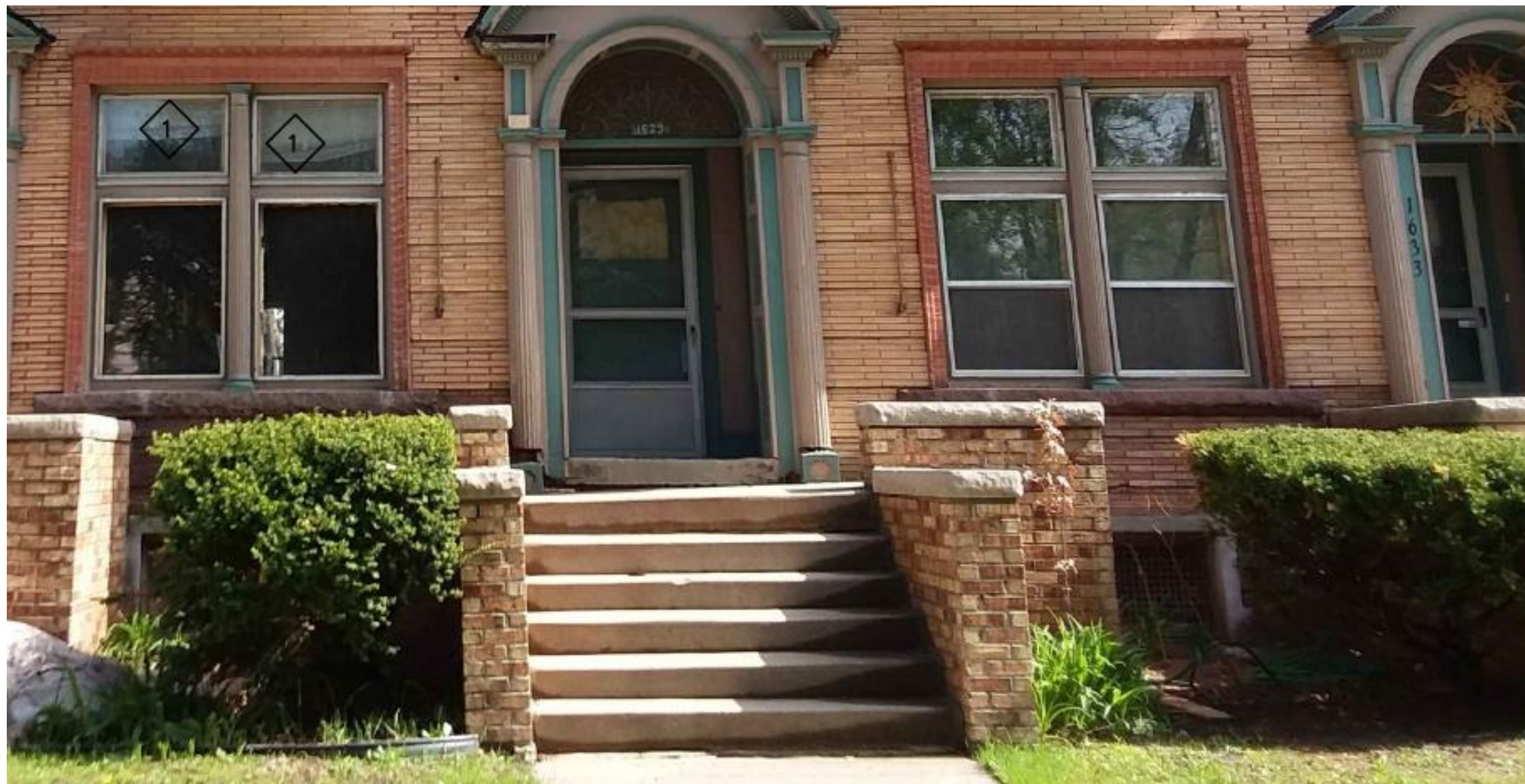
Front elevation porches, prior to unapproved work. Note, pilaster, wood trim, fixed windows and fixed transom
