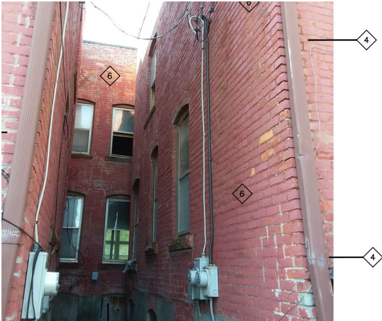
Rear elevation lightwell, prior to unapproved work. Note painted brick
