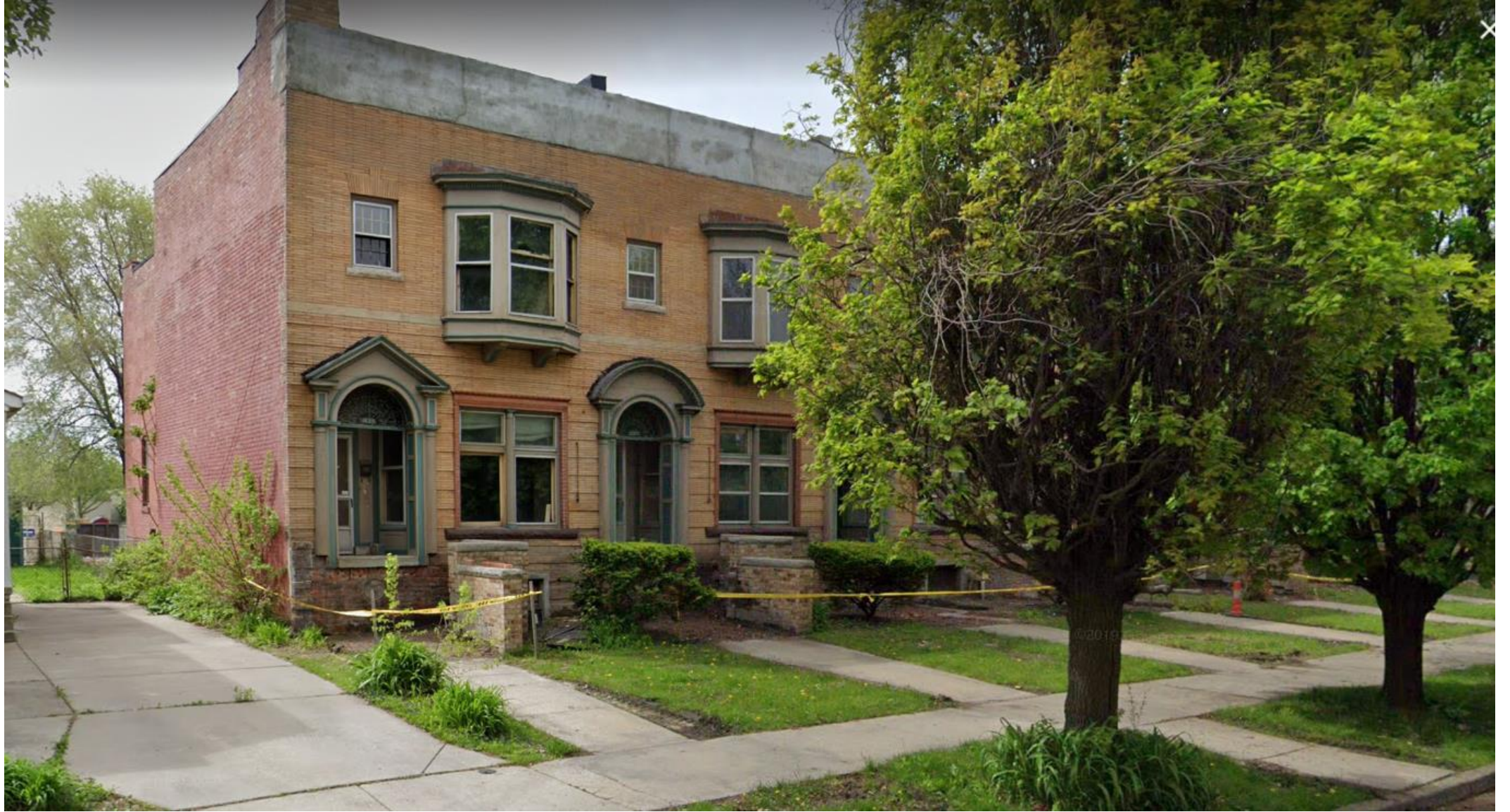
Front elevation, dating from 2019 after the unapproved removal of the original cornice
