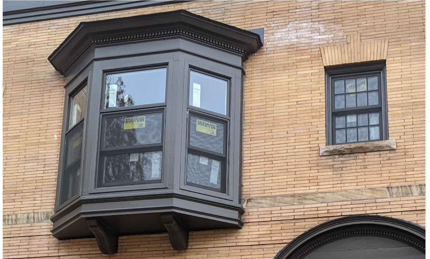
Second-story bay windows current (typical) note 1/1/ windows topped with transom. Also note 8/8 adjacent window
