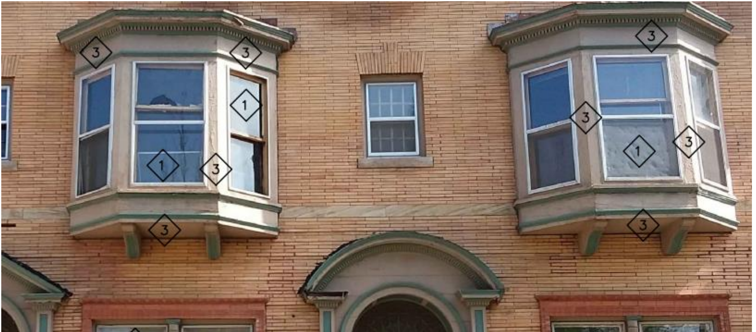
Front elevation window at second story, prior to unapproved work. Note 1/1 and 8/8 wood windows
