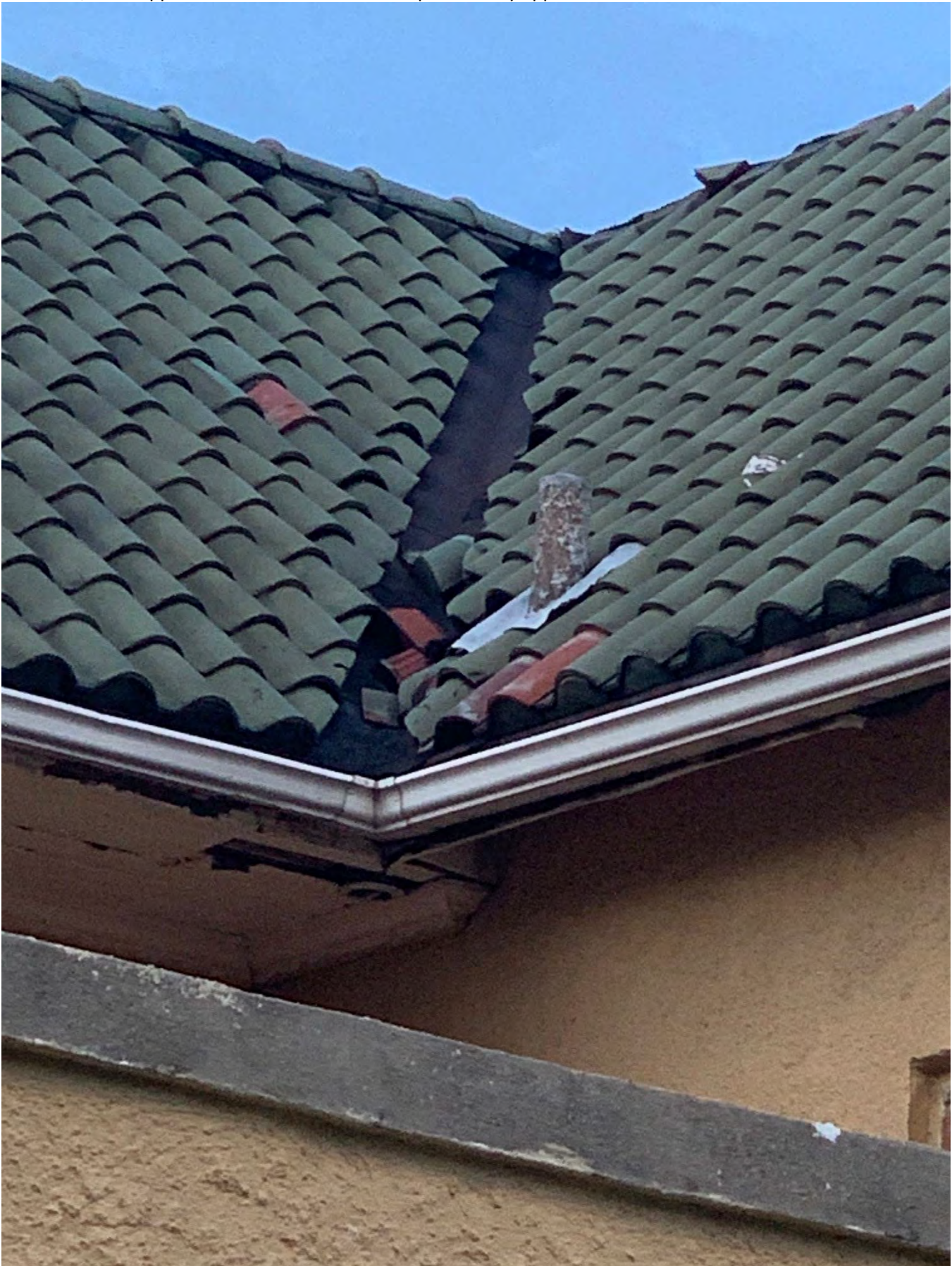
Missing Tile Detail2 9-10
