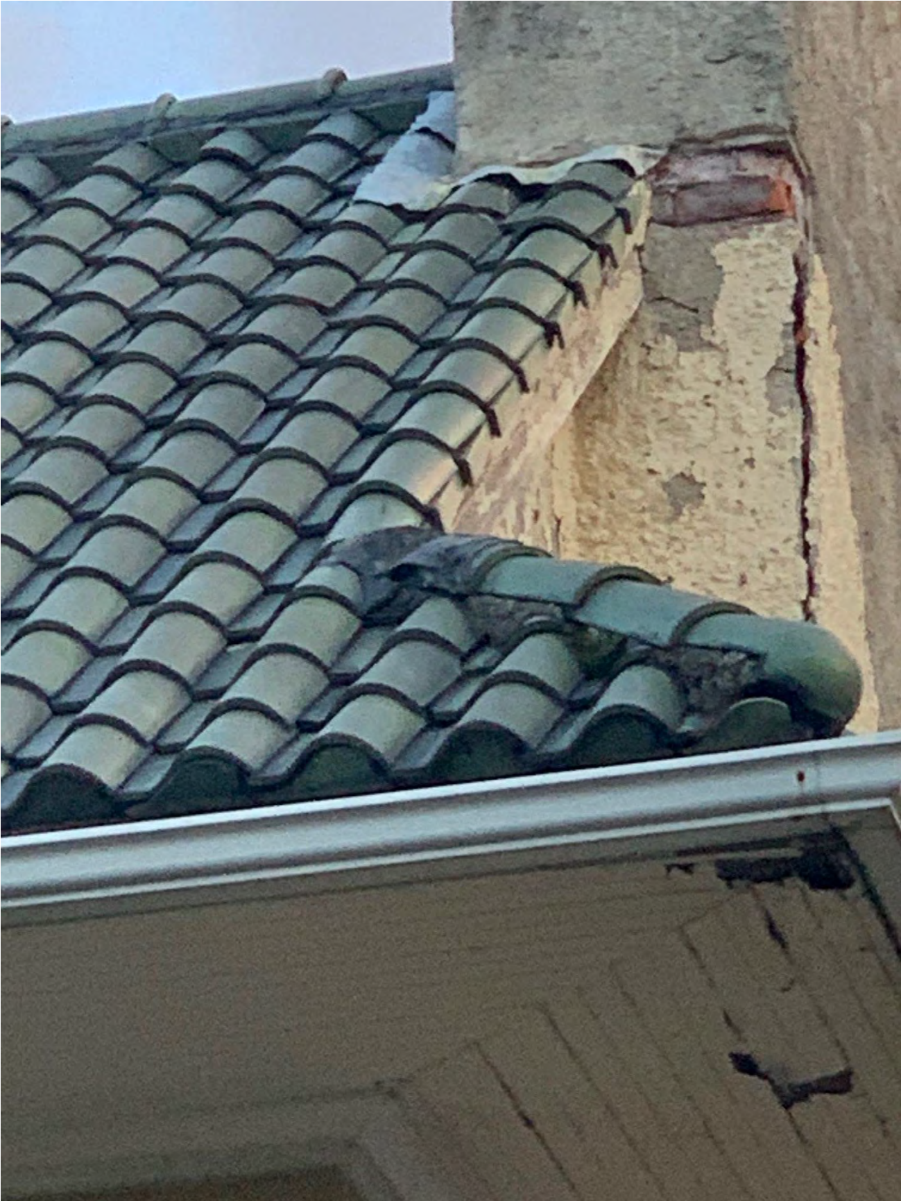
Missing Tile Detail 3 9-10
