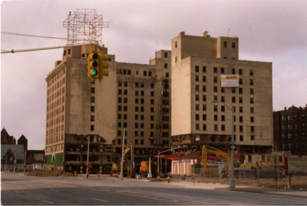
Hotel Detroit, minutes before its implosion in March 1996. It was replaced by low-rise condos along Woodward. HistoricDetroit.org
