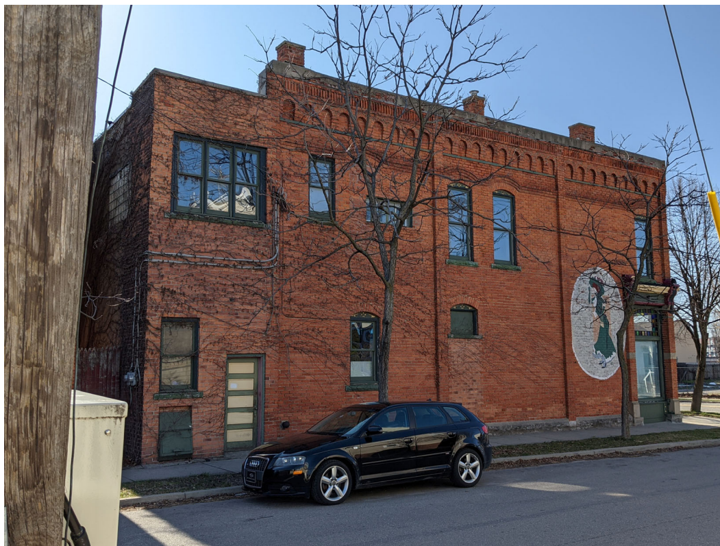
View of existing conditions at 1566 Bagley, view to the east from Tenth. Staff photo, February 26, 2021.
