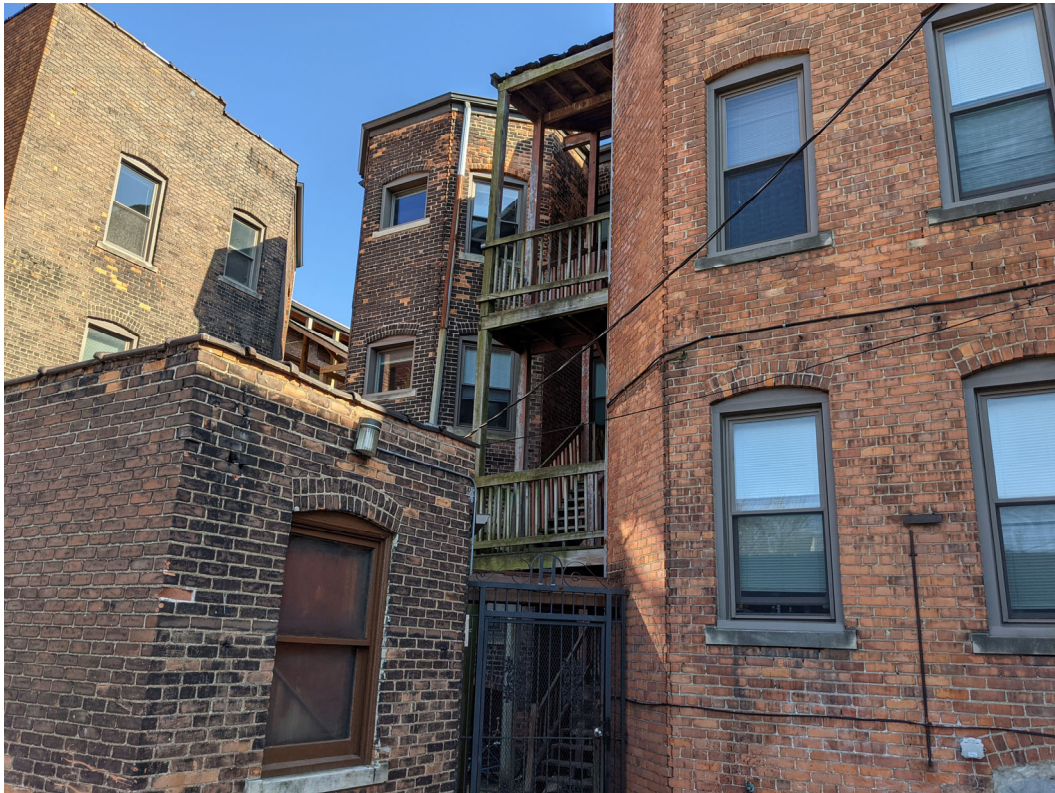
View of existing conditions at rear, showing existing stair. Staff photo, March 29, 2021.
