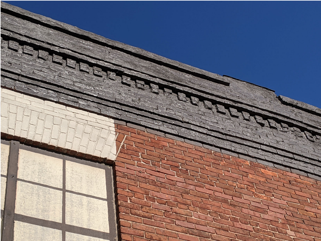
Detail view of parapet at "original" core of the building at Church and 10th. Staff photo, February 26, 2021
