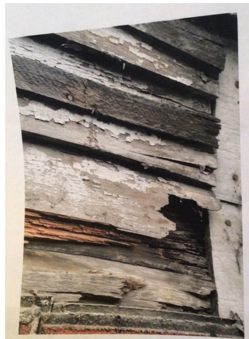
Detail 2 Exposed area under Insul-brick: Applicant Photo
