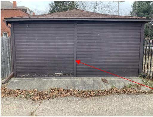
Exterior, north elevation. Proposed location of new garage door. Note, that the vertical element is not structural. It has merely been applied to the exterior wall surface
