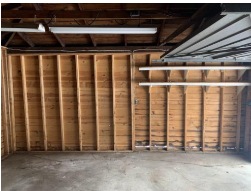
Interior, facing infilled north elevation, proposed location of new door. Note that a center post is not extant.
