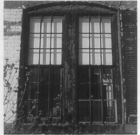
Figure 6. Deteriorating operable windows often contribute to lead dust in a house. Peeling paint and small particles from abraded surfaces collect in window troughs or sills and are then carried inside by air currents, settling on floors. When the lead dust mixes with regular house dust, it can easily be ingested by a child through hand to mouth contact. In homes with small children, floors and other surfaces should be kept as clean as possible to avoid lead contamination.
