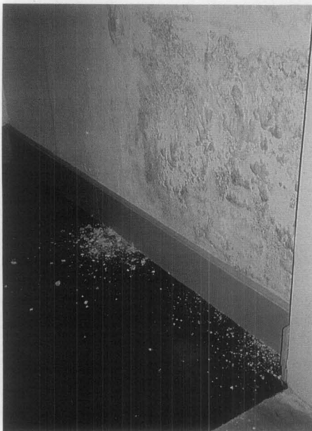
Figure 27. Wall leaks can cause historic surfaces to deteriorate, thereby exposing underlayers of lead-based paint. If painted surfaces show signs of deterioration, they should be repaired as soon as possible.
