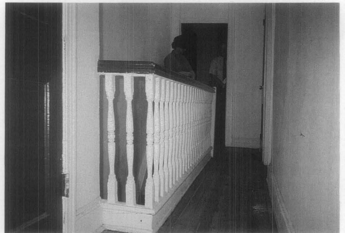
Figure 28. This recently completed housing, which is now lead-safe, could become re-contaminated from lead if safe conditions are not maintained. Damp mopping floor surfaces and regular dusting to keep the house clean will ensure its continuing safety.
