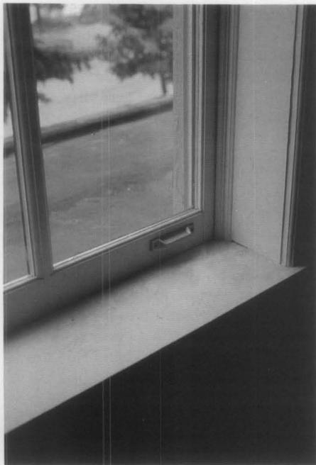
Figure 22. Research has shown that some small children will chew on projecting window sills while teething. As part of a lead hazard control project, the edge of the sill can be stripped to bare wood or an encapsulating paint applied. In this case, a new window sill was installed as part of a window upgrade that retained the historic trim and frame.
