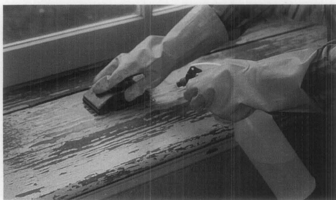
Figure 15. Wet sanding of interior surfaces will keep dust levels down, reduce the need for workers' protection, and provide a sound surface for repainting. Priming and repainting with oil/alkyd, latex or latex acrylic should be undertaken according to manufacturers' instructions.
