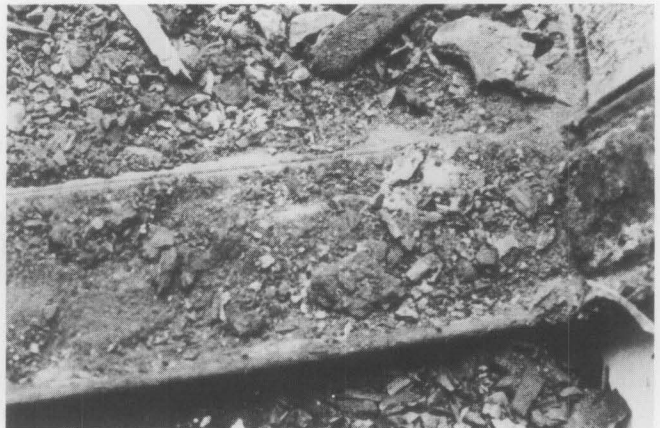
Fig. 6 d. View looking down towards the sill. The subframes appeared very rusted, but were in good condition once debris was vacuumed and surface rust was removed, in place, with chemical compounds. Where necessary, epoxy and steel filler was used to patch depressions in order to make the subframe serviceable again.
