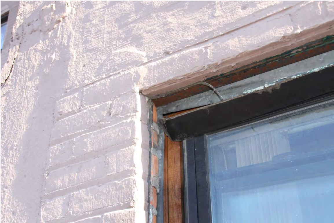
Figure #39: Exterior, Window, Looking Up. 11/18/20
