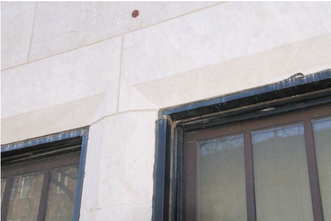
Figure #36: Exterior, Window, Looking Up. 11/18/20
