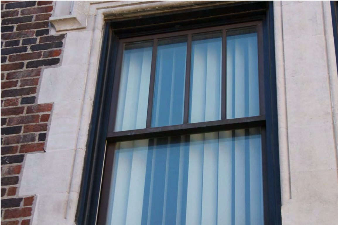
Figure #35: Exterior, Window, Looking Up. 11/18/20
