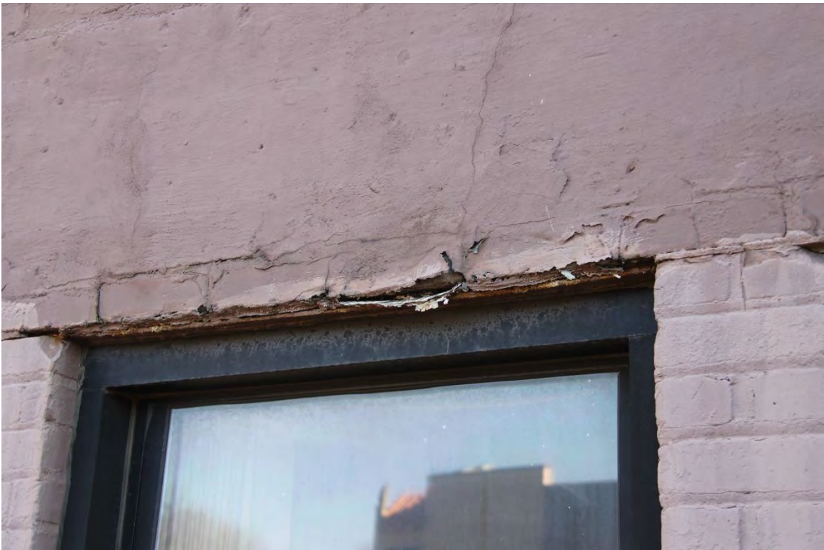
Figure #40: Exterior, Window, Looking Up. 11/18/20
