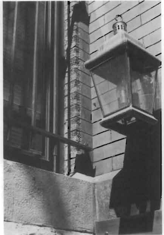
Figure 27. Heavily pitted by sandblasting, this window recess provides a vivid contrast to adjacent undamaged brick protected from abrasion by a metal signboard.
