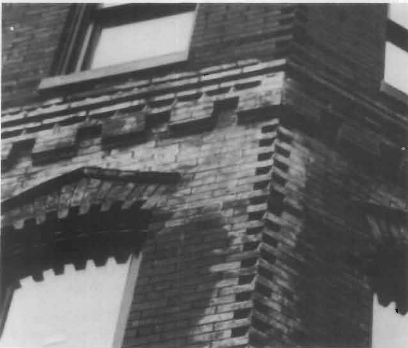
Figure 13. While hydrofluoric acid-based cleaners are often appropriate for cleaning unglazed brick, they may form hard-to-remove whitish silica deposits if left too long on the surface.
