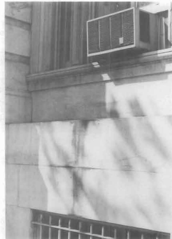
Figure 22. The discoloration on this white marble is a green-colored algae growth on a shady side of the building and caused by water dripping from the air-conditioner above it.
