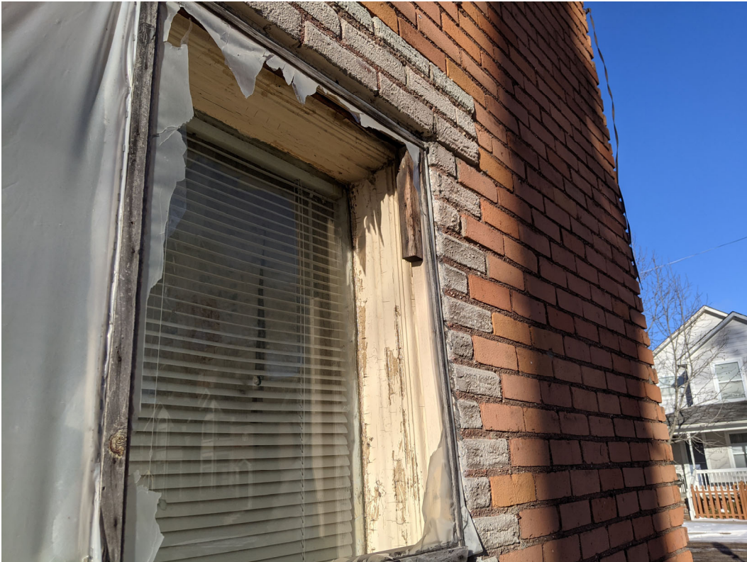
Detail view of shop window frame at first story along Brooklyn Street. Staff photo, February 3, 2021.
