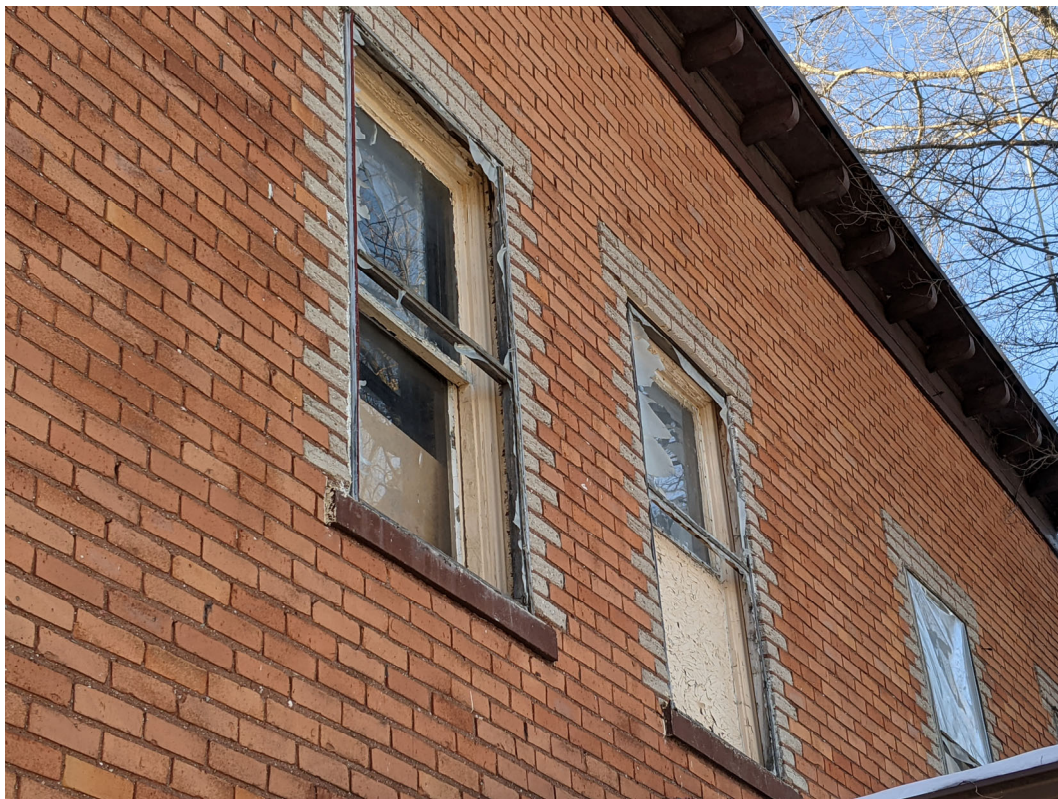
Detail view of windows at second floor. Though there are many areas requiring paint and repair, with certain elements missing and/or requiring replacement, the work would not be technically challenging. Staff photo, February 3, 2021.
