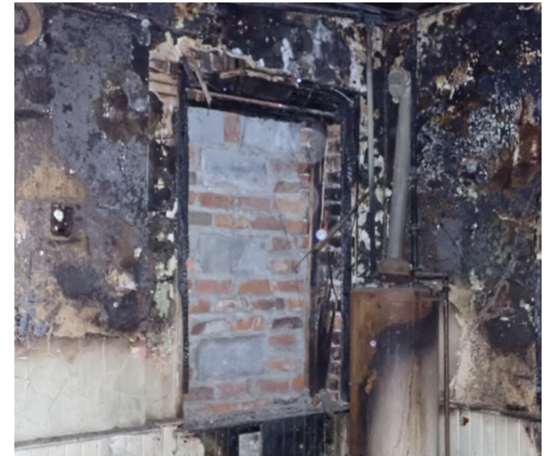
UNIT 208: FIRE DAMAGE
