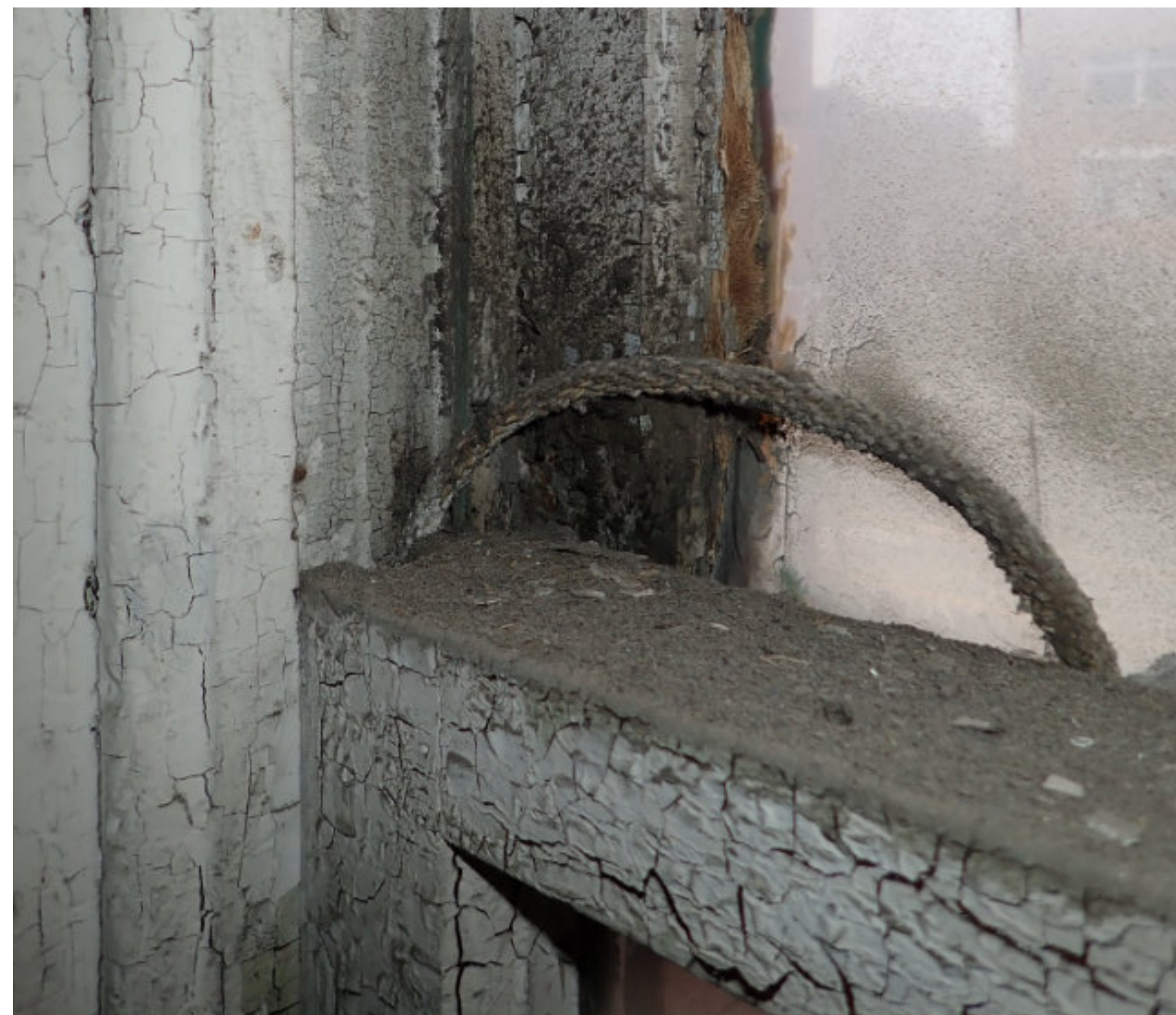
UNIT 206: BROKEN ROPES AND ANCHORS
