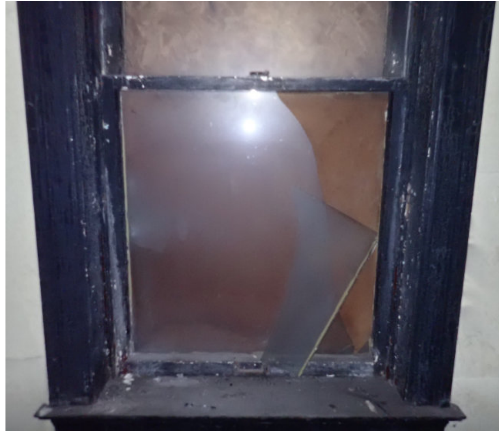
UNIT 201: BROKEN GLASS IN WINDOW FRAME
