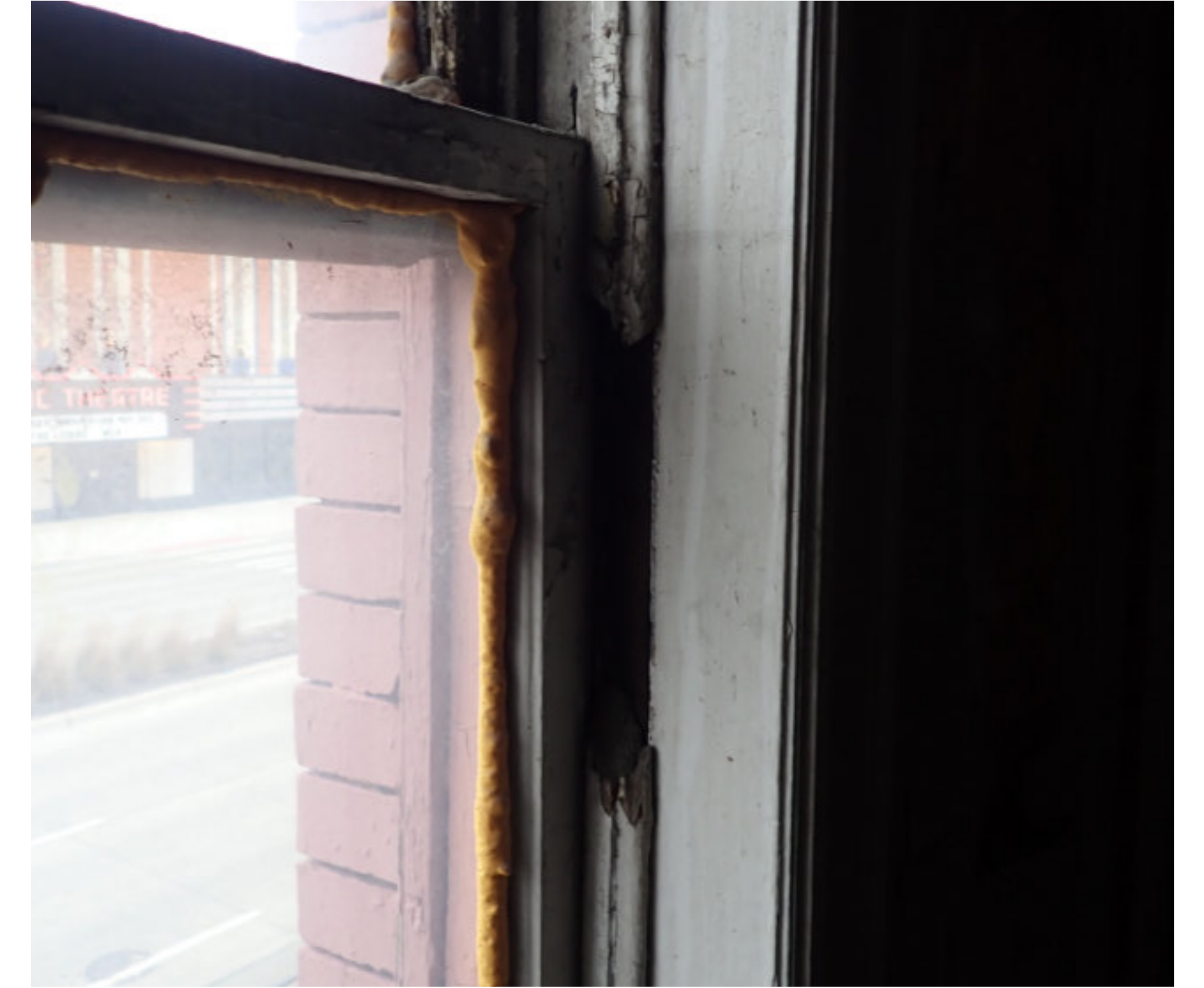
UNIT 207: BROKEN AND MISSING STOP
