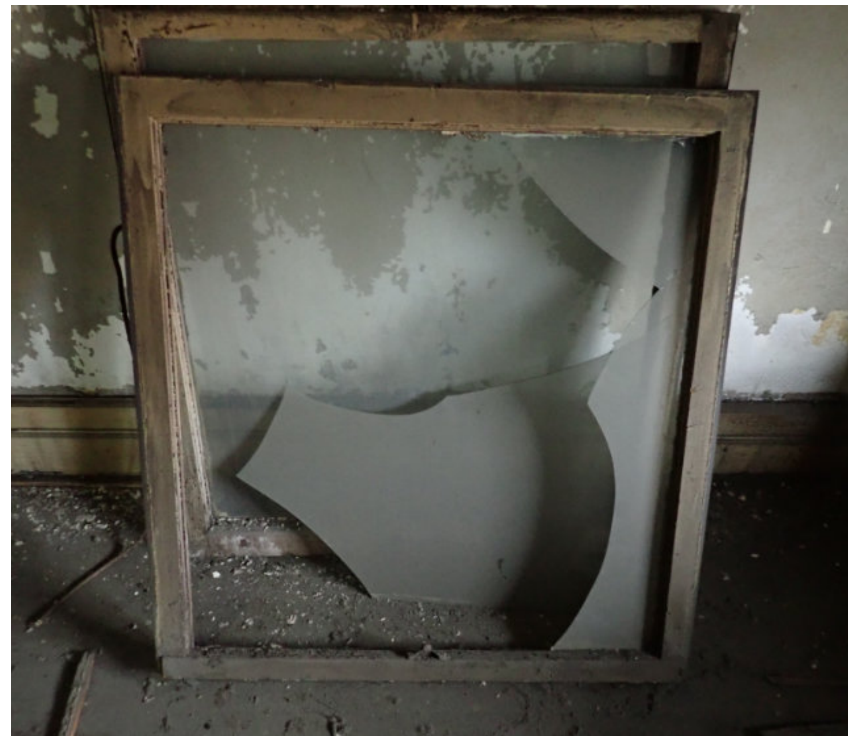
UNIT 204: REMOVED FRAMES WITH BROKEN GLASS
