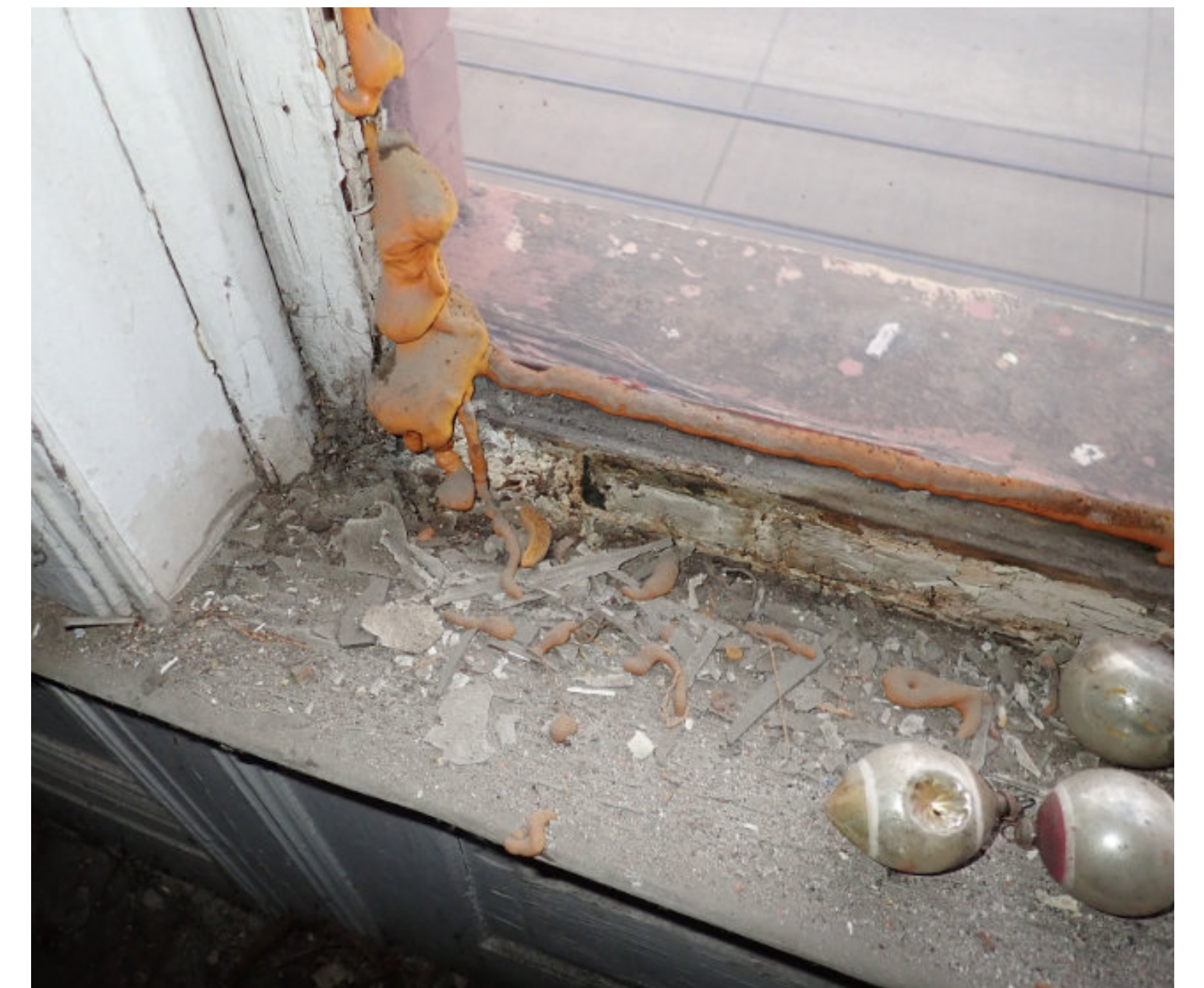
UNIT 207: INAPPROPRIATE MATERIAL
