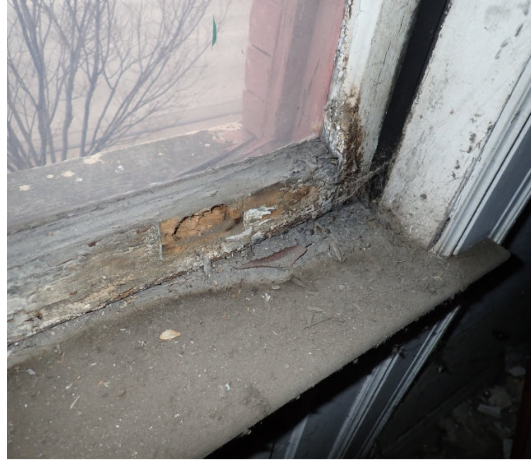
UNIT 206: DETERIORATED LOWER RAIL
