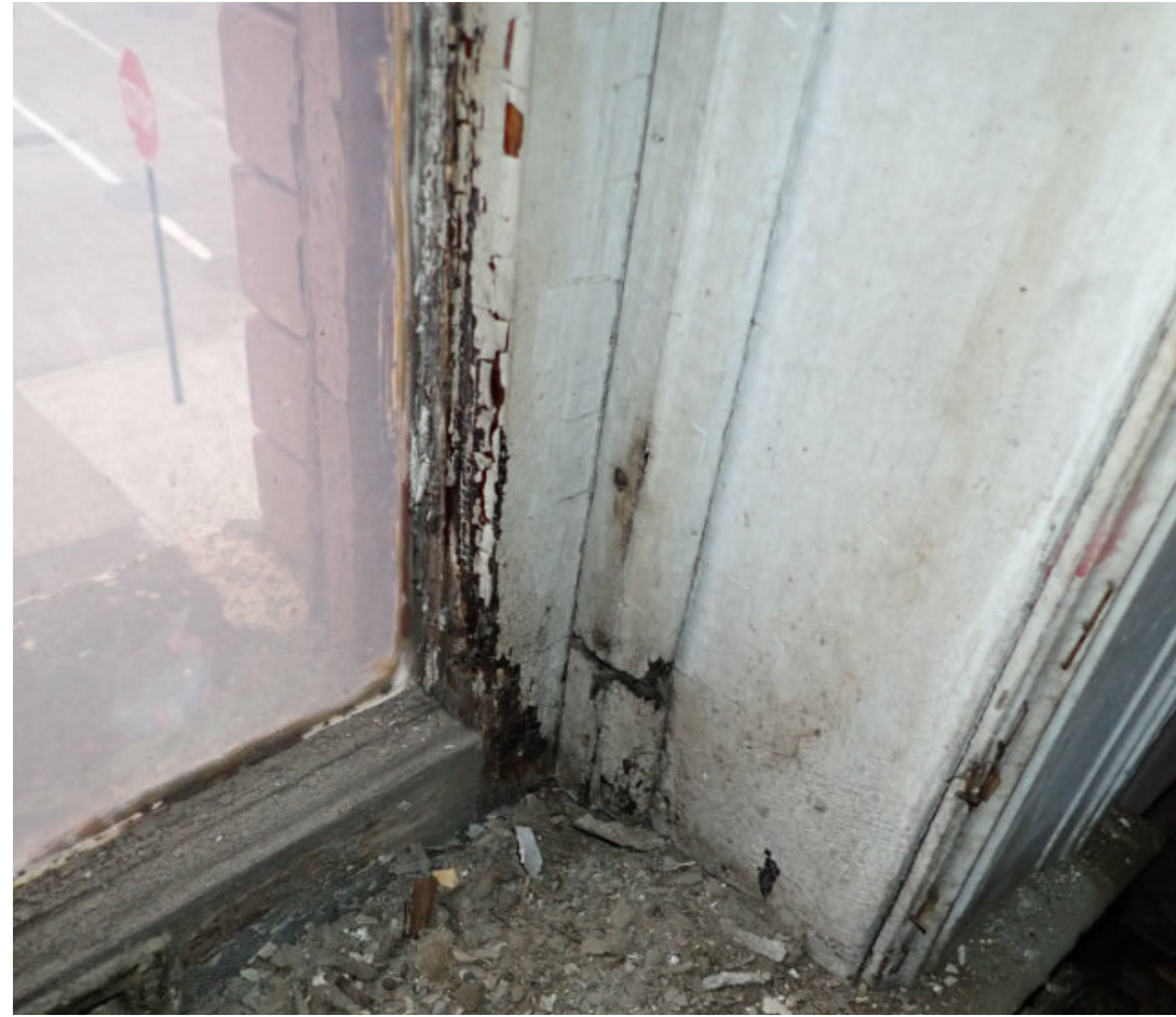
UNIT 208: DETERIORATED STILE
