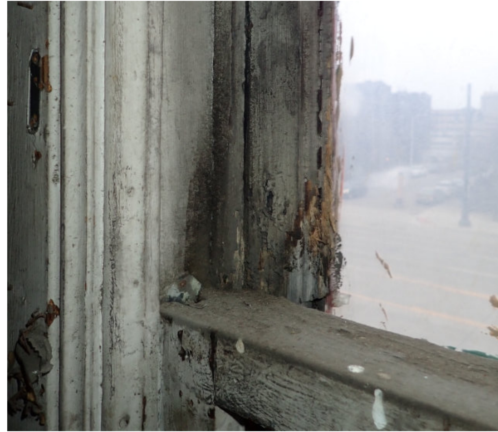
UNIT 208: DETERIORATED STILE
