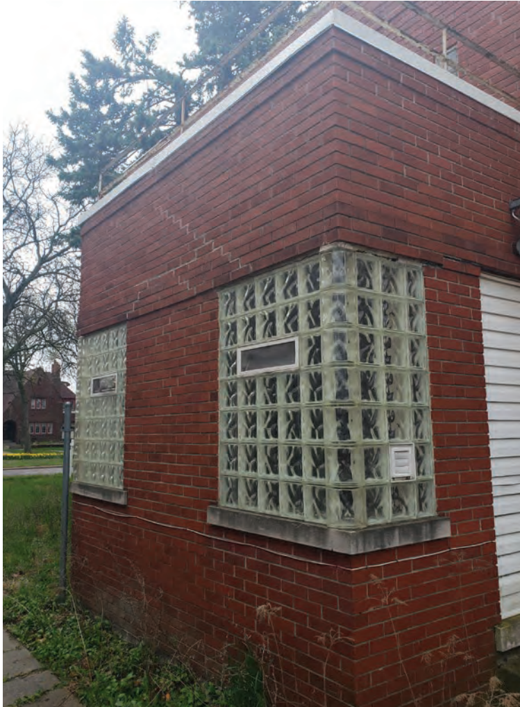
Fig. 3A | Today, the windows have been replaced with glass block. See window type (W-3) for more informaton
