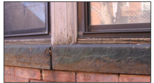
1 st floor window, viewable sill condition - poor
