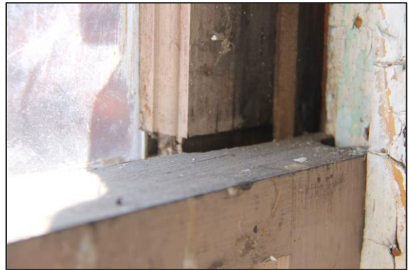
Failed Sash Joinery
