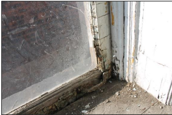
Failed Corner Joinery, Bottom Rail
