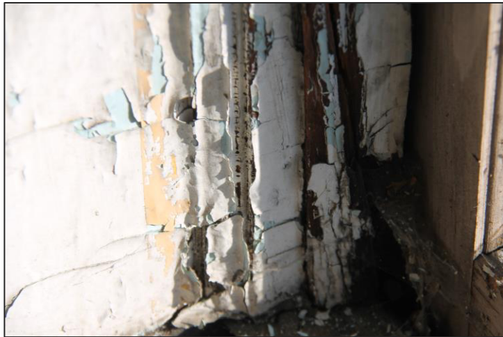
Rotted jamb behind board-up that was removed
